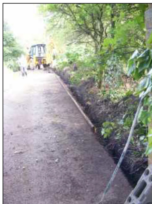
Plate 3: Working shot during the machining of the new service trench in Area C, looking N.
