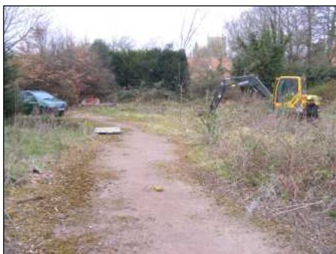
Plate 2 (left): Area A2 at the start of machine excavation, looking W towards the church.
