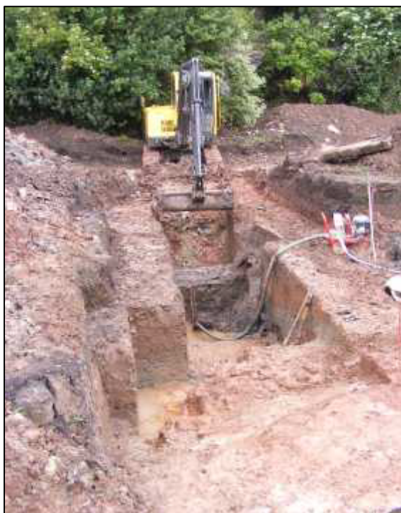
Plate 17: Working shot excavating a full profile through the 'channel' in Area A2, recorded as section 474. Looking north-east.
