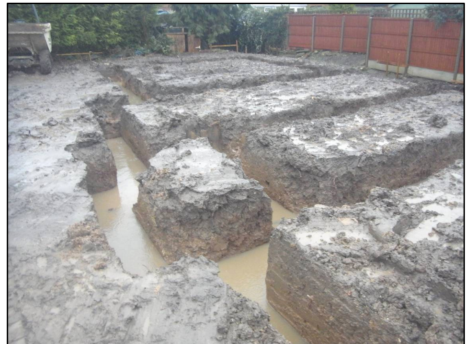
Plate 4: The completed footings trenches of the house plot, showing the ground conditions during the project.
