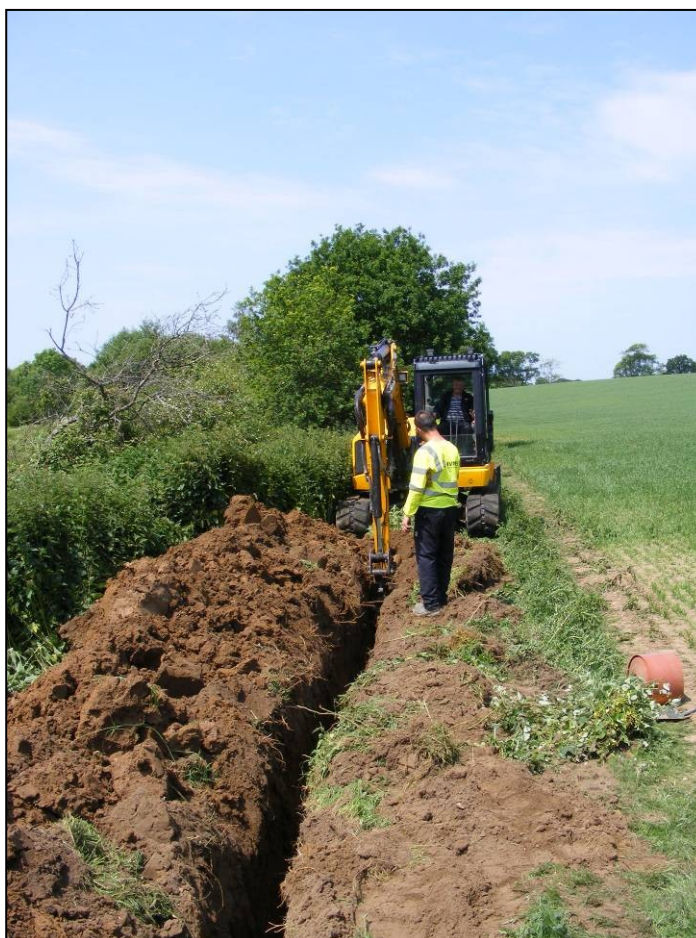
Plate 1: Working shot of second leg of the southern cable route, looking west.
