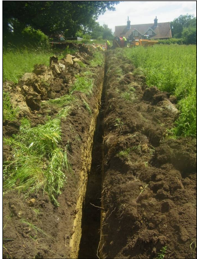
Plate 4: Looking east along the east-west leg of the northern cable route, towards the houses on the western periphery of Albourne
