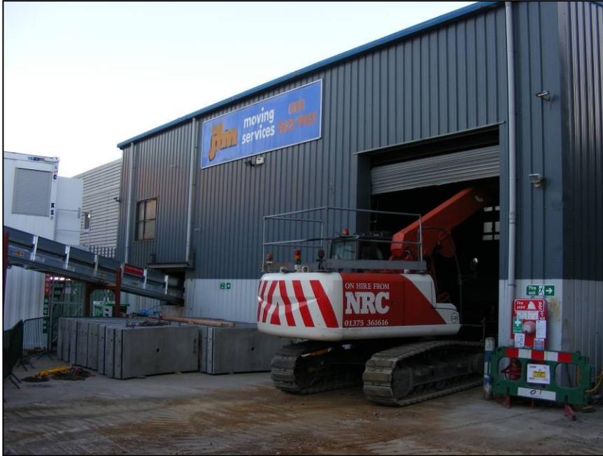
Plate 1: Industrial unit at the time of archaeological monitoring. Access shaft is excavated within the shell of the building.
