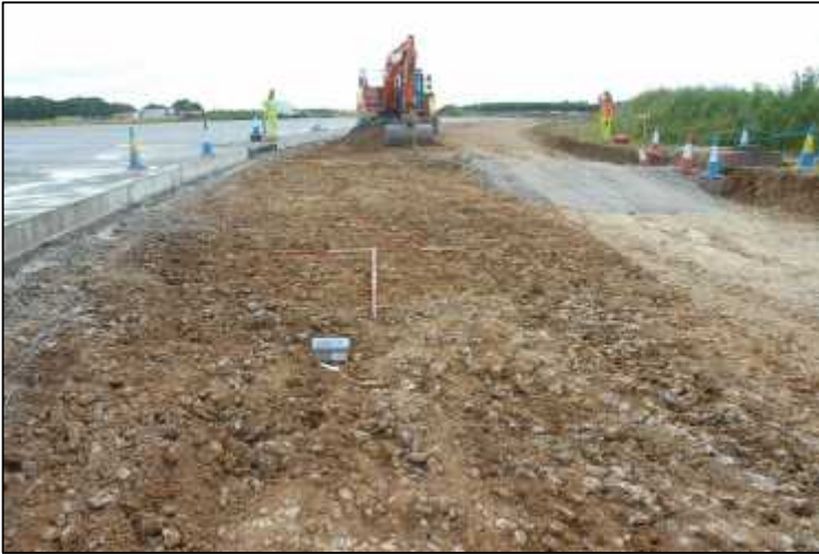
Plate 3: Excavation at the north side of the taxiway, looking southwest, showing the natural stone.
