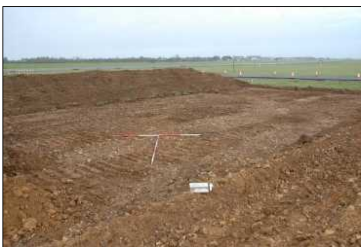
Plate 2: Topsoil strip at the beginning of groundworks on the taxiway, looking north. The break in the line of trees on the horizon, almost directly on the line of the north arrow, shows the course of Roman Ermine Street. The abundant stone in the topsoil strip proved on deeper excavation to be natural in origin.
