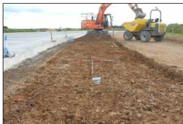
Plate 1: Working shot of the strip along the north side of the existing runway, looking south-west.
