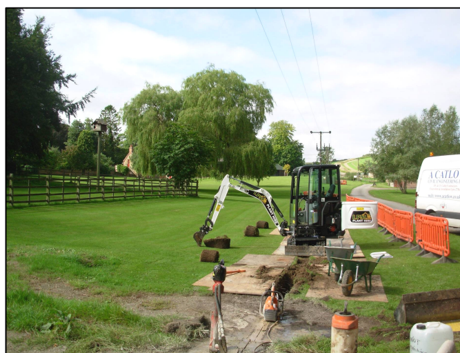
Plate 4: Working shot during trench excavation along the road, looking west-north-west from the area of concrete hard-standing.
