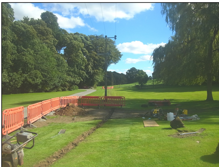
Plate 5: The excavated cable trench, looking east from a point a short distance to the west of Test Pit 2.
