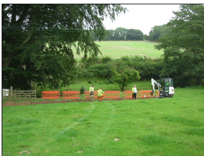
Plate 3: Working shot during trenching into the field, looking north-east: the trees to the rear mark the course of the Waithe Beck.
