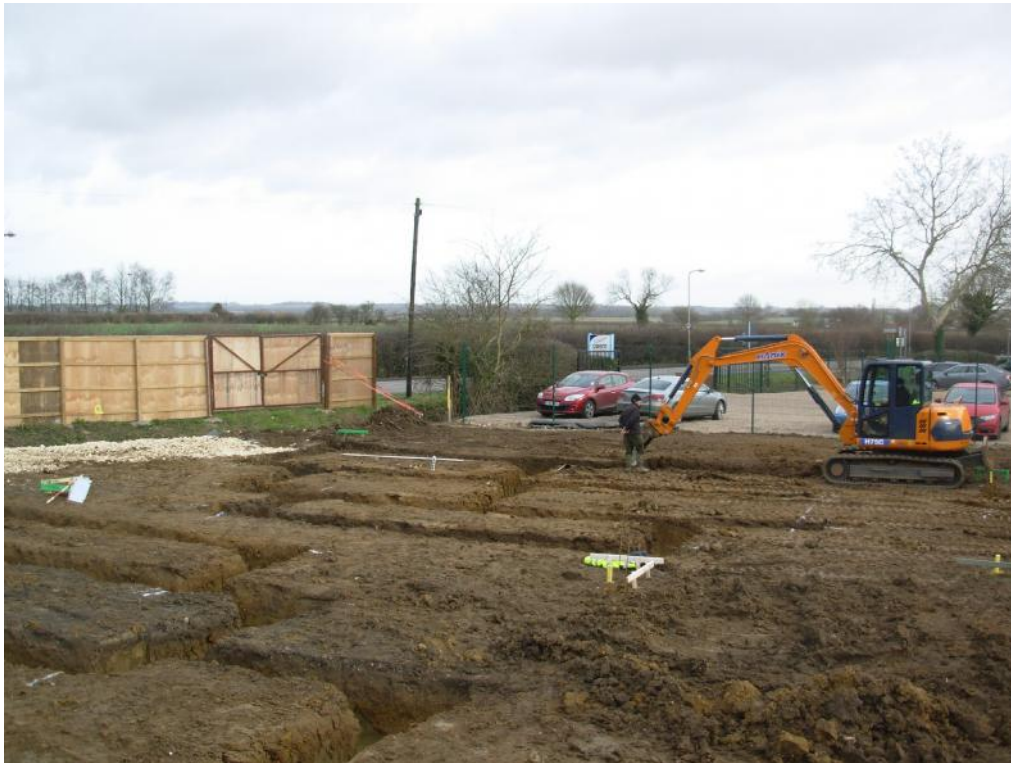
Plate 2: Site after topsoil strip and during excavation of footing trenches, facing north-east
