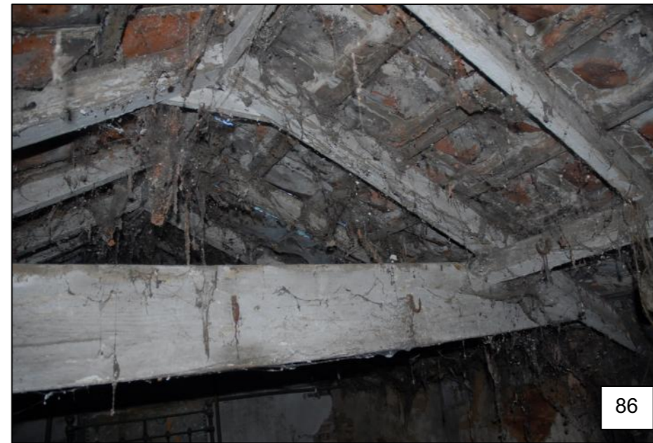
The collar-principal rafter roof has clasped through-purlins, ridge collars and a ridgeboard.
