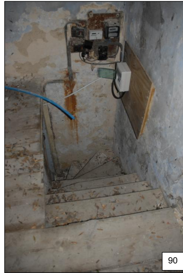
The winding timber staircase rises from Room 7 rises in the northeast corner (rear stairs: go 9¼", rise 9¼"; and wind to east and south), but has no safety rail. The room is whitewashed throughout.
