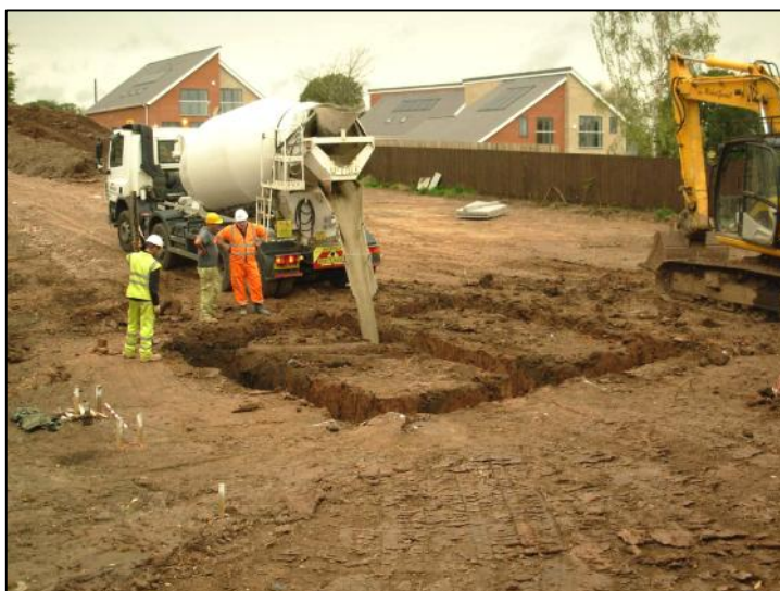
Plate 4: The completed garage footings at the end of the first day, looking north-west.
