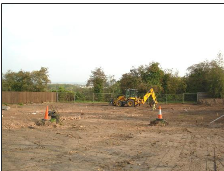
Plate 2: General shot of the area of monitoring during machining, looking ENE, showing the topography of the lower end of the site.
