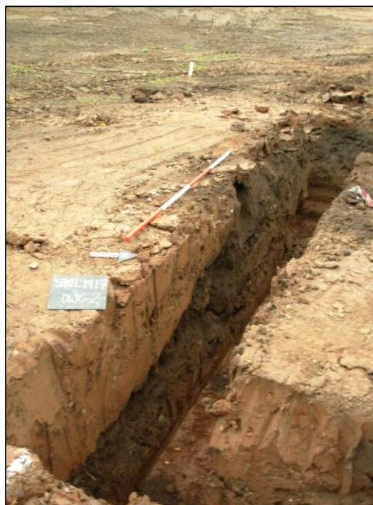
Plate 3: North-facing section of the garage footings, looking south-west, showing the modern infill of the canal and the dark layer of topsoil that had previously accumulated on the sides of the empty canal bed.
