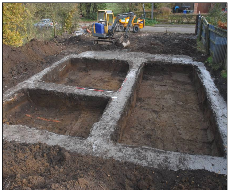
Plate 2: The completed building plot footings after the removal of material from between them, looking east north east.
