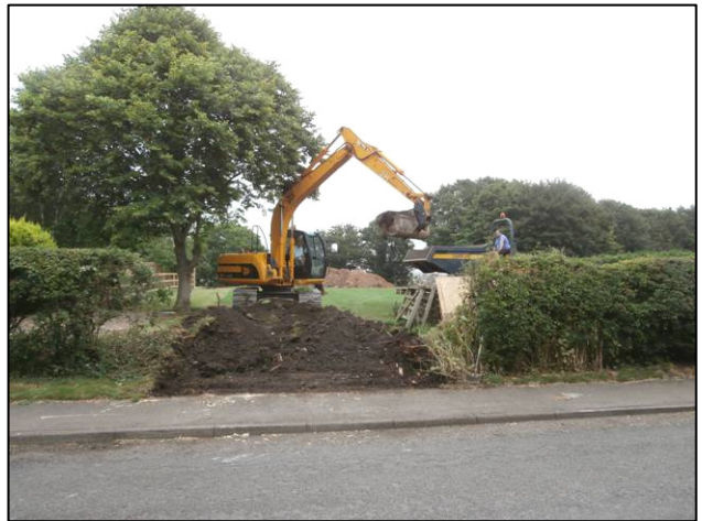
Plate 3: Working shot at the start of construction works, looking NE from the far side of Main Street during groundworks for the new drive.
