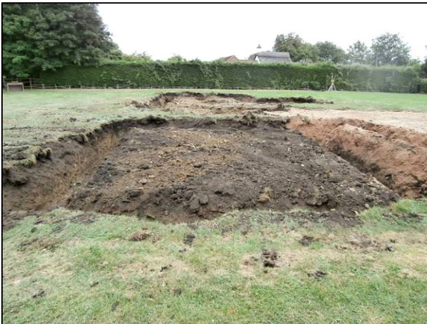
Plate 4: The completed foundation trenching, looking ESE with the garage in the foreground and the house in the background.
