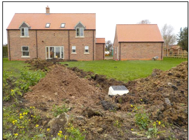
Plate 5: The drainage works, completed after the construction of the house and garage, looking S from the location of the bio-treatment unit pit.
