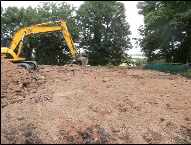
Plate 2: Working shot during the removal of the tennis court, looking NE: the position of the site at the top of a north-facing slope, looking out over the river valley, can be seen.
