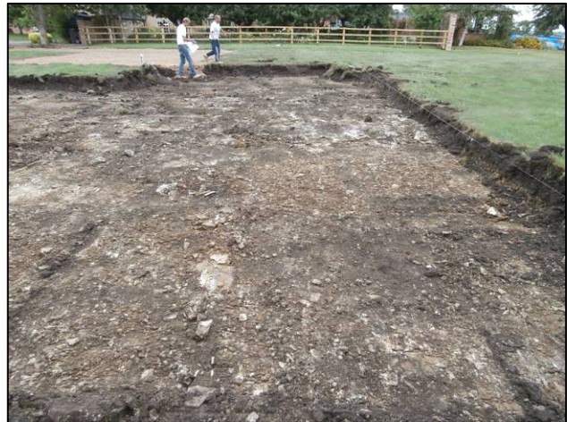
Plate 5: The house footprint stripped to the surface of the natural, looking NW.
