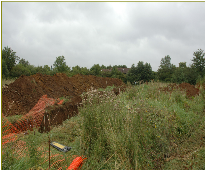
Plate 4: Trench 2, looking north-east. The site was overgrown with high grass and weeds. The height of the site is demonstrated by the level relative to the roof tops in the distance.
