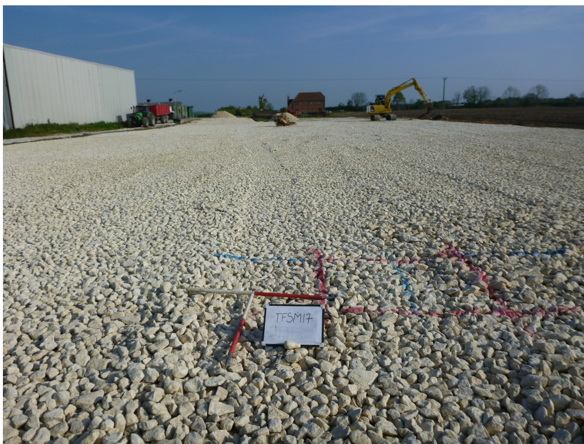
Plate 1: General view of development area prior to excavation of base pads (looking NNW)
