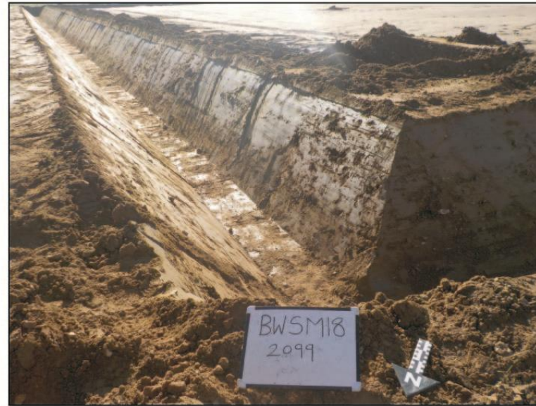
Plate.8: Looking south at spill drainage syatem at the Well Site
