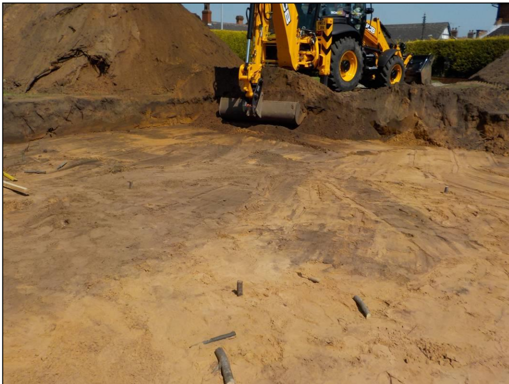
Above: Topsoil and subsoil were removed separately before ground level reduction. Looking ENE
