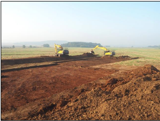
Plate 3: Machine top- and subsoil stripping in Area 4, following the line of the pit alignment, looking south-west.
