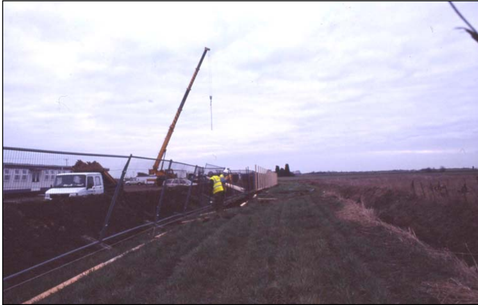
Plate 5: General view showing the hand excavation of the post holes for the wooden hoarding fence looking south
