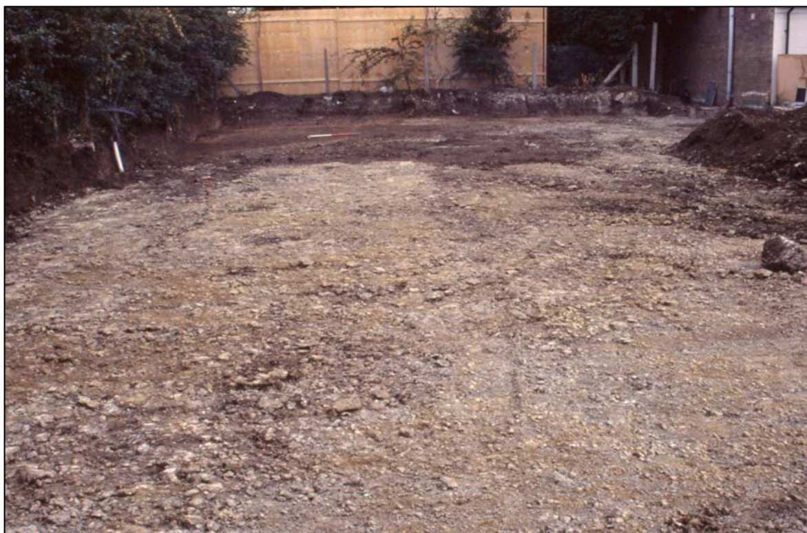
Plate 2: Rear of site showing concentration of earth-cut features (dark areas), looking east.
