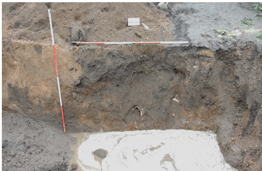
Plate 9: Northwest limit of pipe trench showing service trench [314] that appears to run under the standing cross.
