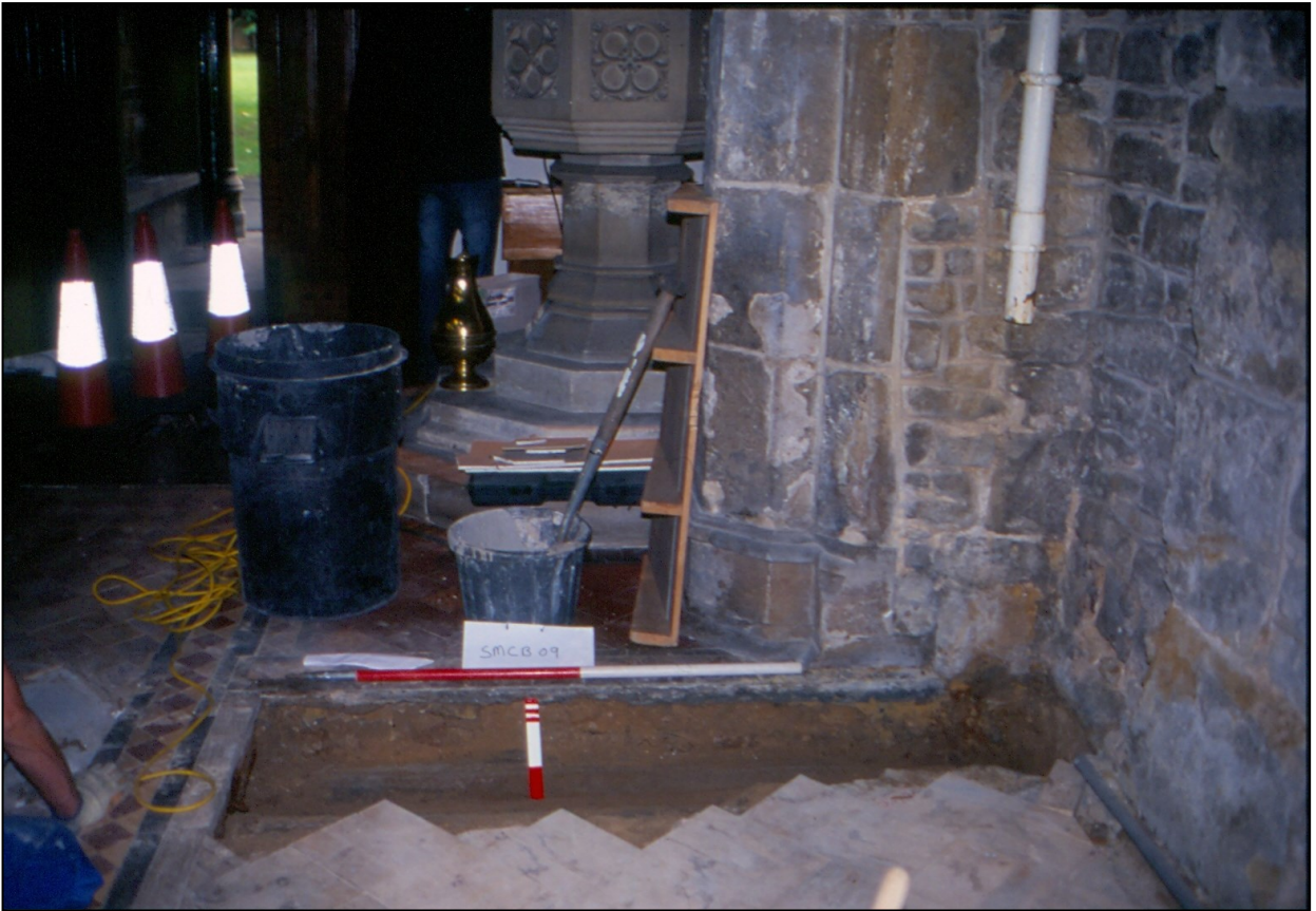
Pl. 1 Position of the monitored pipe duct (looking south towards the porch, with the east wall of the tower in the foreground, right. Scales 2m and 0.25m).
