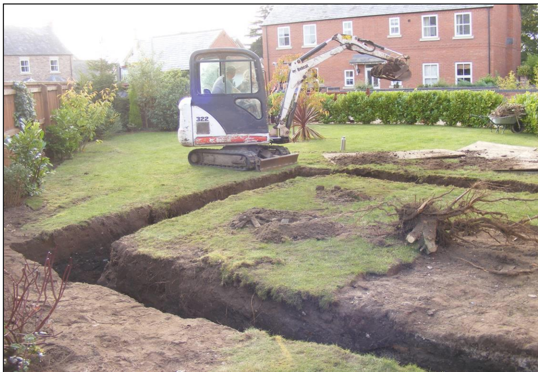
PI. 2 Footprint of the new extension (looking south-west towards No. 1 Abbey Park).
