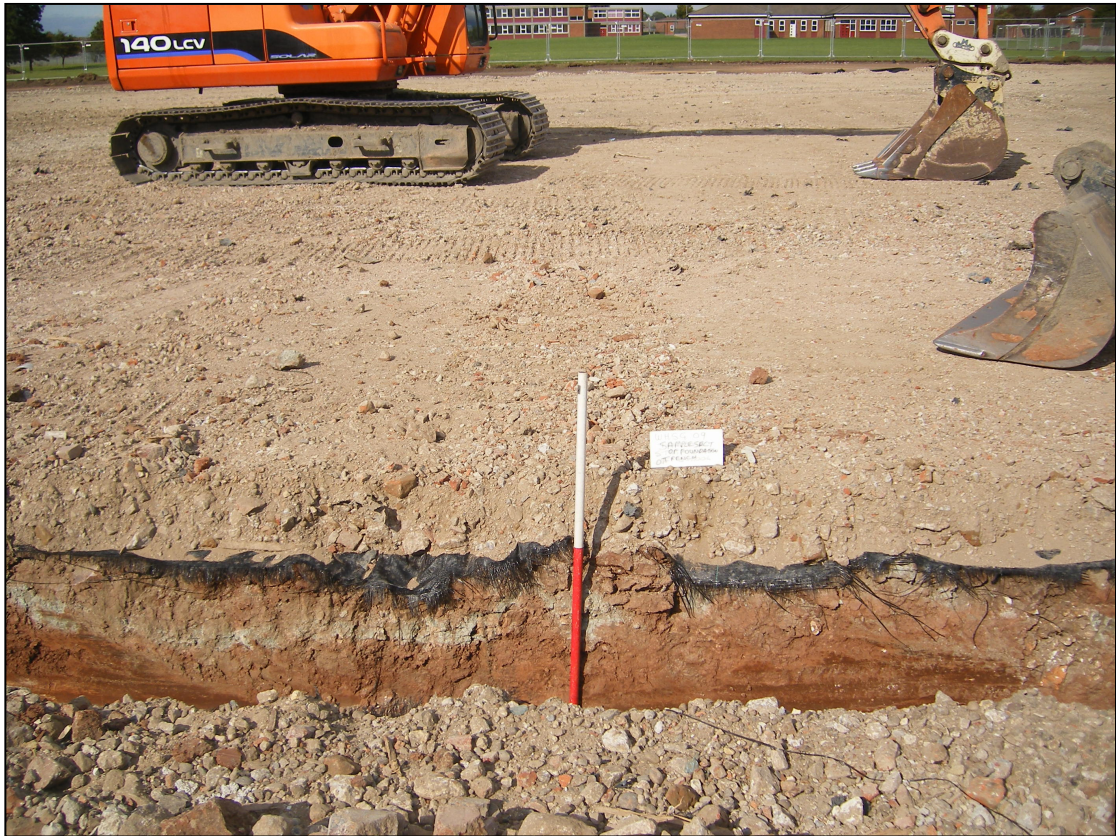
Pl. 7 A terram membrane was laid over the stripped area, and this was covered with crushed hardcore. The foundation trenches for the new school buildings were excavated from this level, only revealing undisturbed natural clay (looking north, scale 1m).
