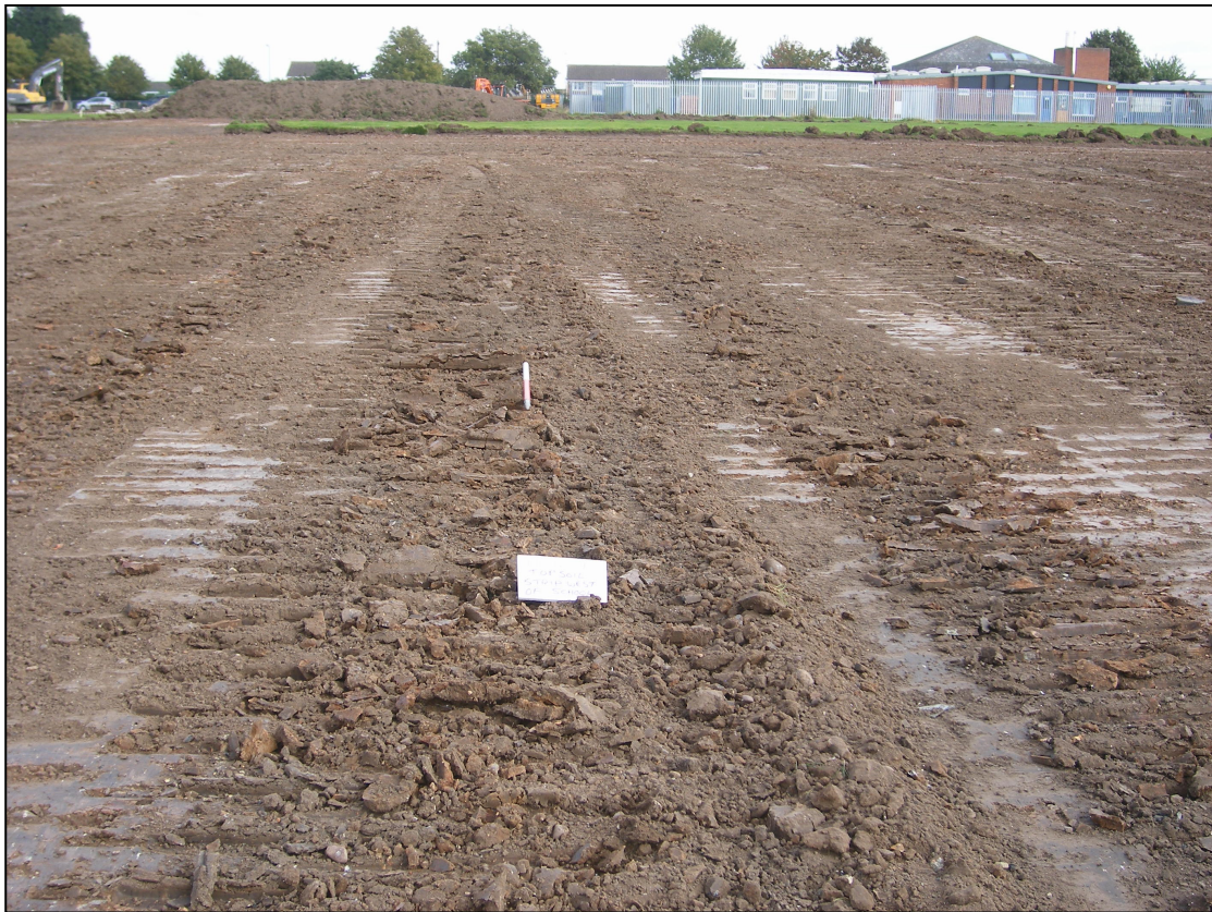
Pl. 6 Detail of the surface left after topsoil removal (looking south towards the existing school buildings).
