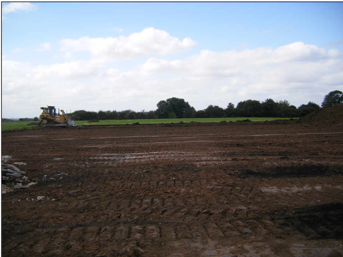
Pl. 4 The stripped surface was trampled and disturbed by the machine tracks and was not in suitable condition for the identification of archaeological features (looking west).
