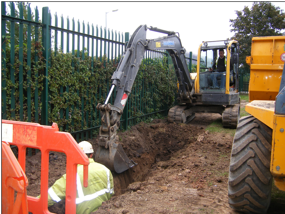
Pl. 8 Excavation of the sewer trench alongside the Middlefield Lane boundary (looking south).
