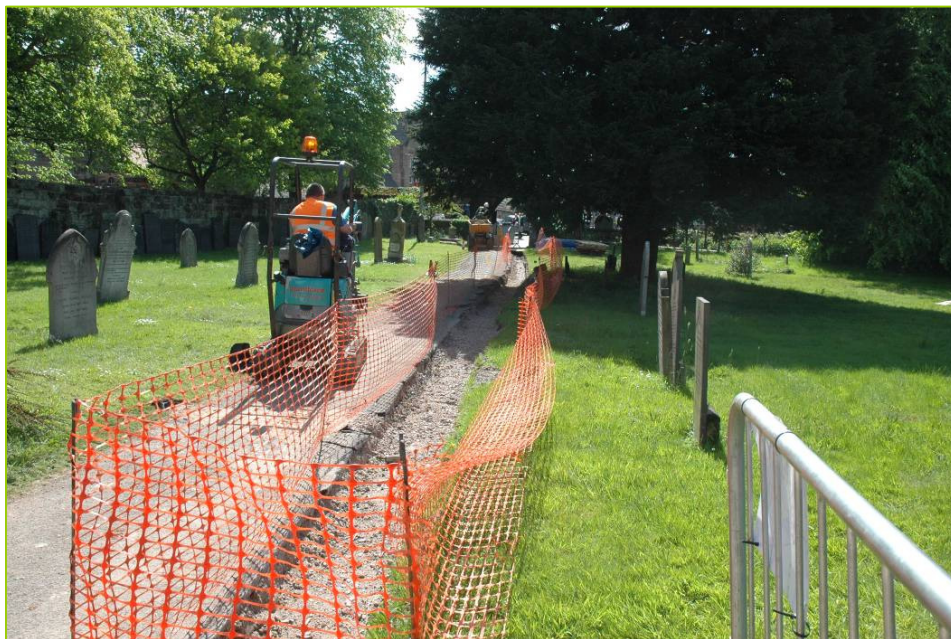
PI. 8 External pipe trench to the west of the church (looking west).
