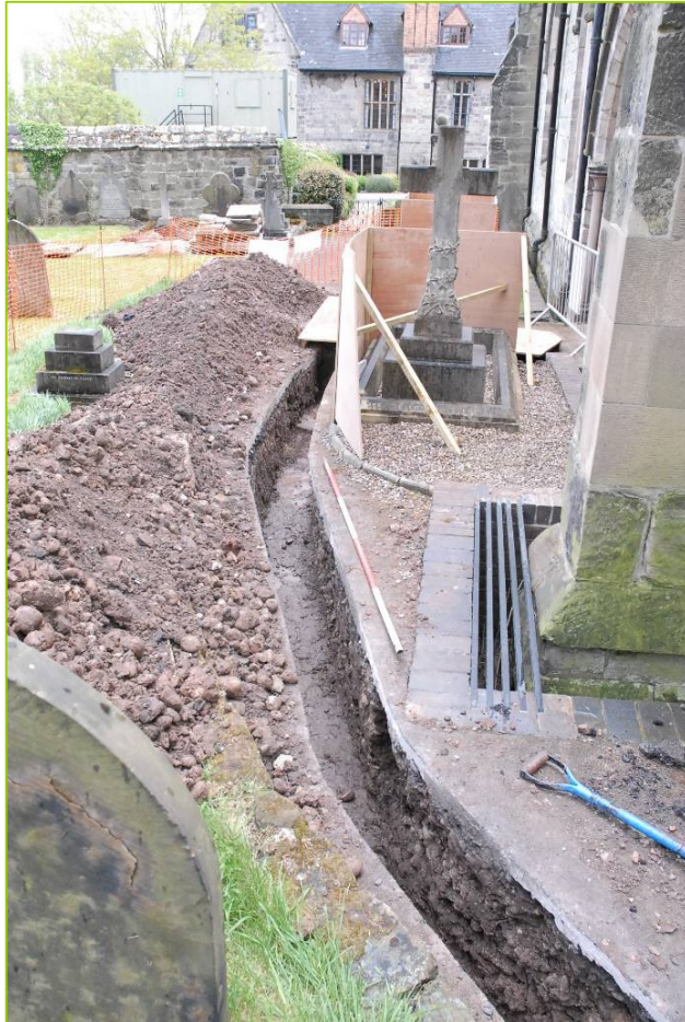
PI. 7 External pipe trench, to the north-west of the church (looking east, scale 2m).
