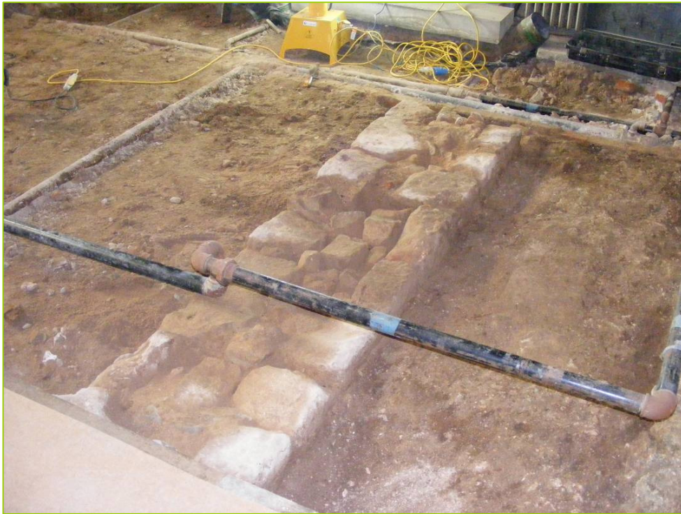
PI. 1 Outer vestry works following the removal of the floor surfaces and some underlying deposits. Wall (109) can clearly be seen as can the system of pipes that disturbed the area (looking south-west).
