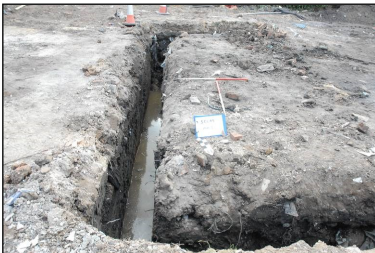
Plate 2: Plot 1. Foundation trench, (Frame 15) looking south, showing modern rubbish pit in foreground.
