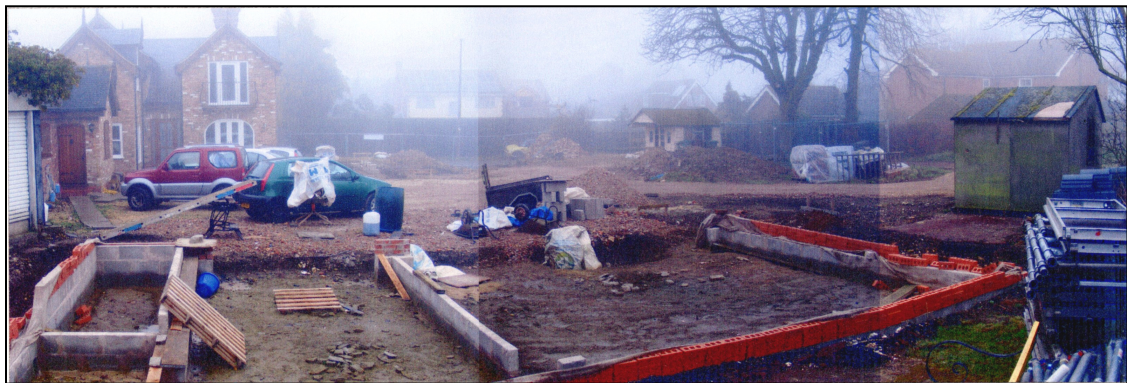
Plate 2: Composite shot of the site before trenching began, looking north towards Post Office Lane across the foundations of the new garage building.
