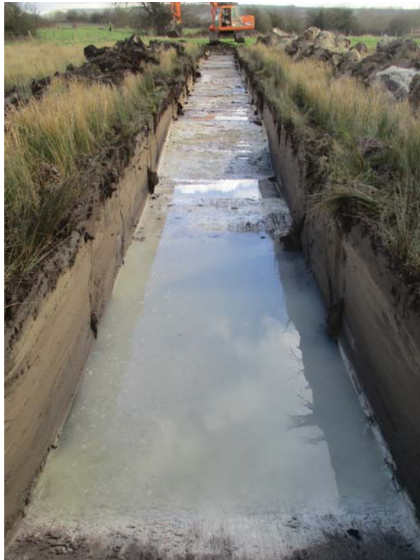
View of Trench 3 immediately after machining, ditch 308 and pit 318 are below the water in the foreground
