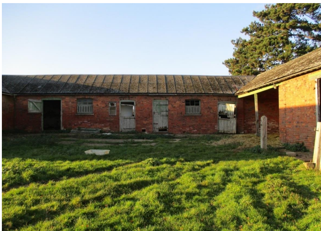
Photo 8: Cattle yard and south-east facing elevation of central range. The surface area nearest to this range is laid with concrete, which has since broken up.
