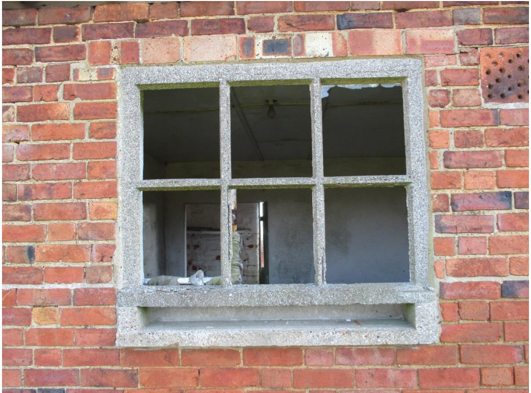
Photo 15: Concrete window-frame, inserted at a later point to increase light into the building. Note also the earlier clay ventilation panel at upper-right.
