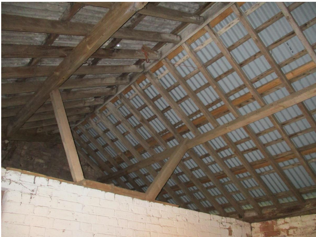
Photo 10: Roofing within central range. This is the earlier timber structure as first constructed. The struts support purlins, which in turn carry common rafters.
