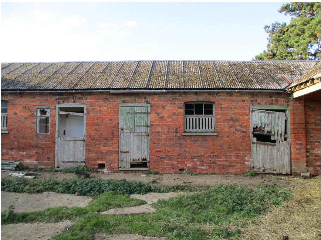
Photo 14: Central range with doors into rooms 4-6. Note the window, with ventilation slits to the lower part and what was originally six-light glazing to the upper. These have been repaired and reworked. Guttering is asbestos.
