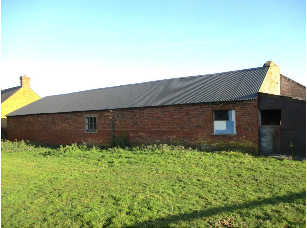
Photo 3: Rear elevation of cow house, looking south-east. The metal roof is later.
