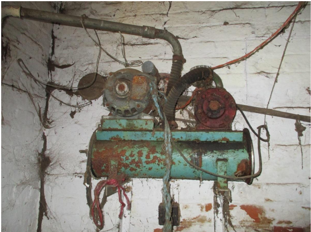
Photo 20: Small pump engine in room 6.
