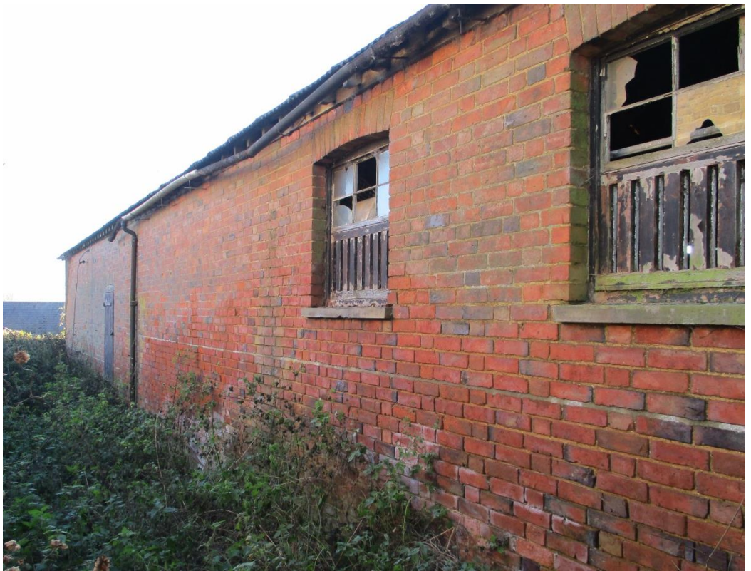
Photo 4: North-east facing elevation facing. Note the ventilation slits to windows. Note the mix of guttering and downpipes: cast-iron and asbestos.
