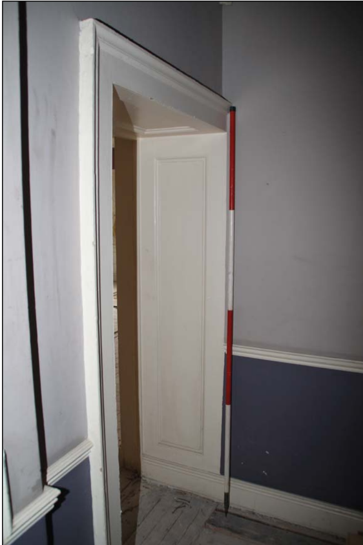
The south-east reveal of the door from 1.2 into 1.1. The skirting and dado on the right are later 20th century fittings around the stair enclosure. On the left is the mid 19th century dado (scale in 0.5m divisions)
