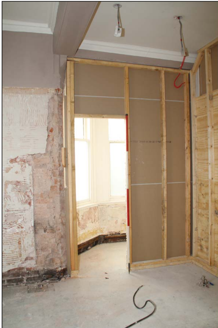
The bay window off 1.6, looking west with corniced beam where was once a wall and modern stud work going in (scale 2m)
