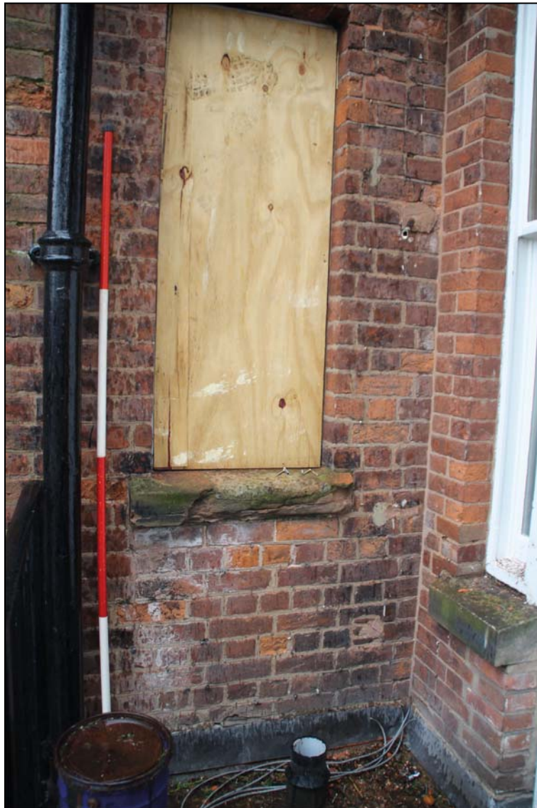
The unbonded internal corner of the Friary and Bird Street ranges showing different brick sizes and bonds (scale 2m)
