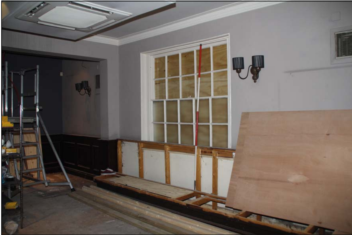
Room G7 to G8 and the large sash window in the south-west wall (scale 2m)
