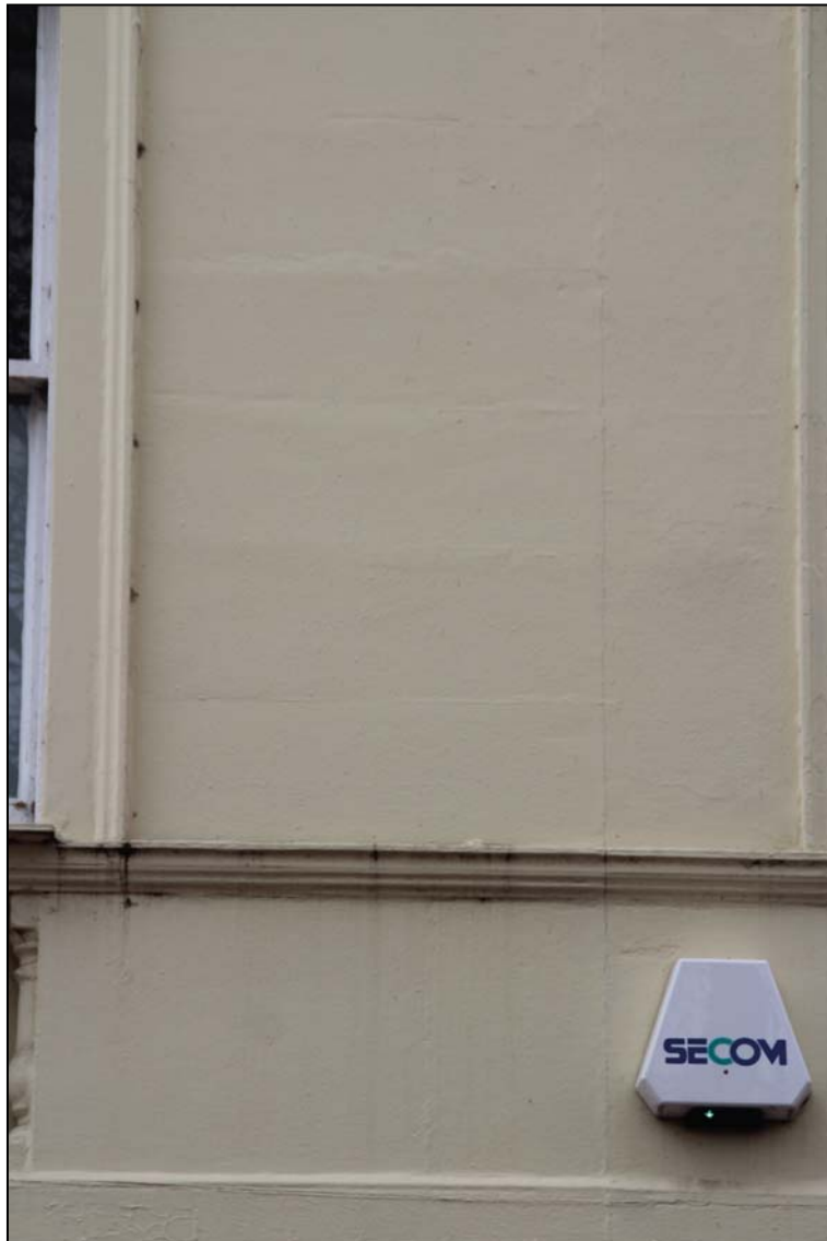
The junction of the painted ashlar facing on the Friary range with the painted render on the Bird Street block
