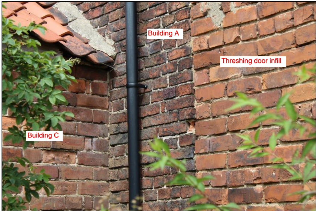
Photo 32: Detail of junction between eastern elevation of Building C and southern elevation of Building A
