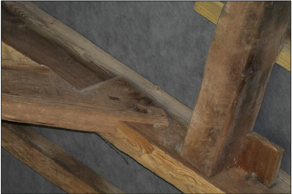
Photo 17: Detail of half-dovetail lap joint between collar and rafter of truss II
