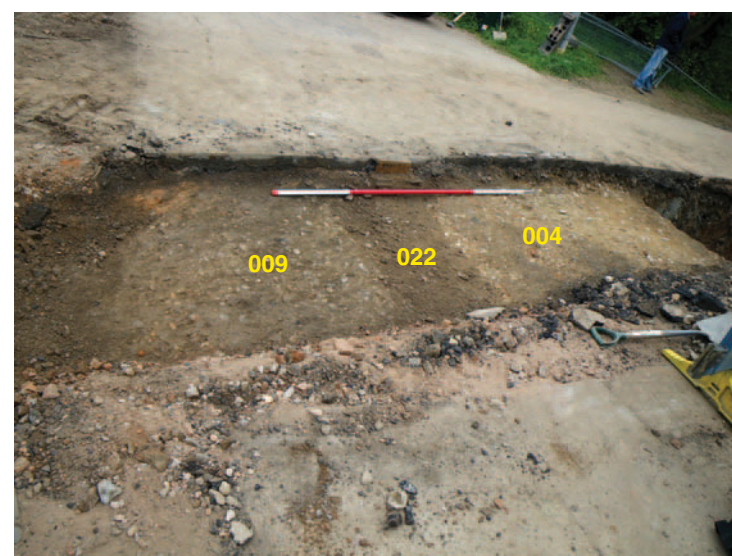
The exposed road metalling 004/009, looking north-east, camber evident on left, gas main 022 visible in centre under scale. Scale 2m
