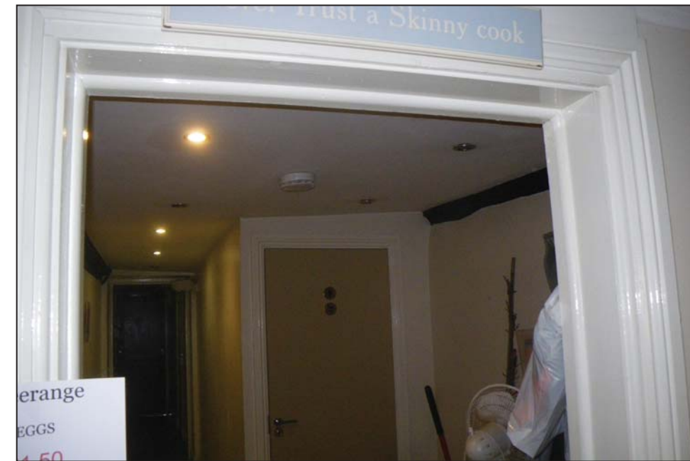
9 In the cafe rear corridor (Block 3a) looking to the south-east showing beams at ceiling level
