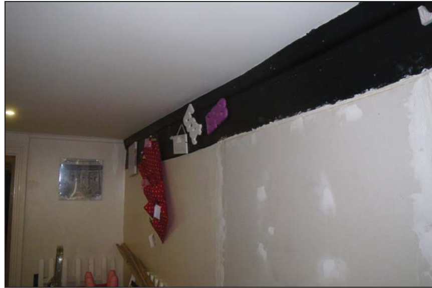
12 Inside the cafe entrance (Block 3a) looking to the south-east showing the beam at ceiling level in the party wall and blocked door below
