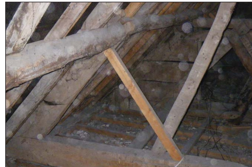
15 One of the phase 3 trusses, showing butt purlins and tie beam. Phases 1 and 2 visible at rear
