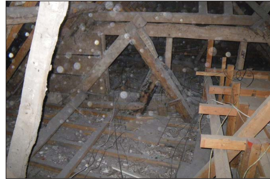
14 The roughly built extension of Phase 2, looking north-west. The north-west building's hipped gable end is evident immediately behind it
