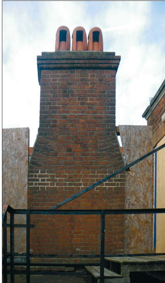
7 The chimney stack on the south end of the west wing, looking north
