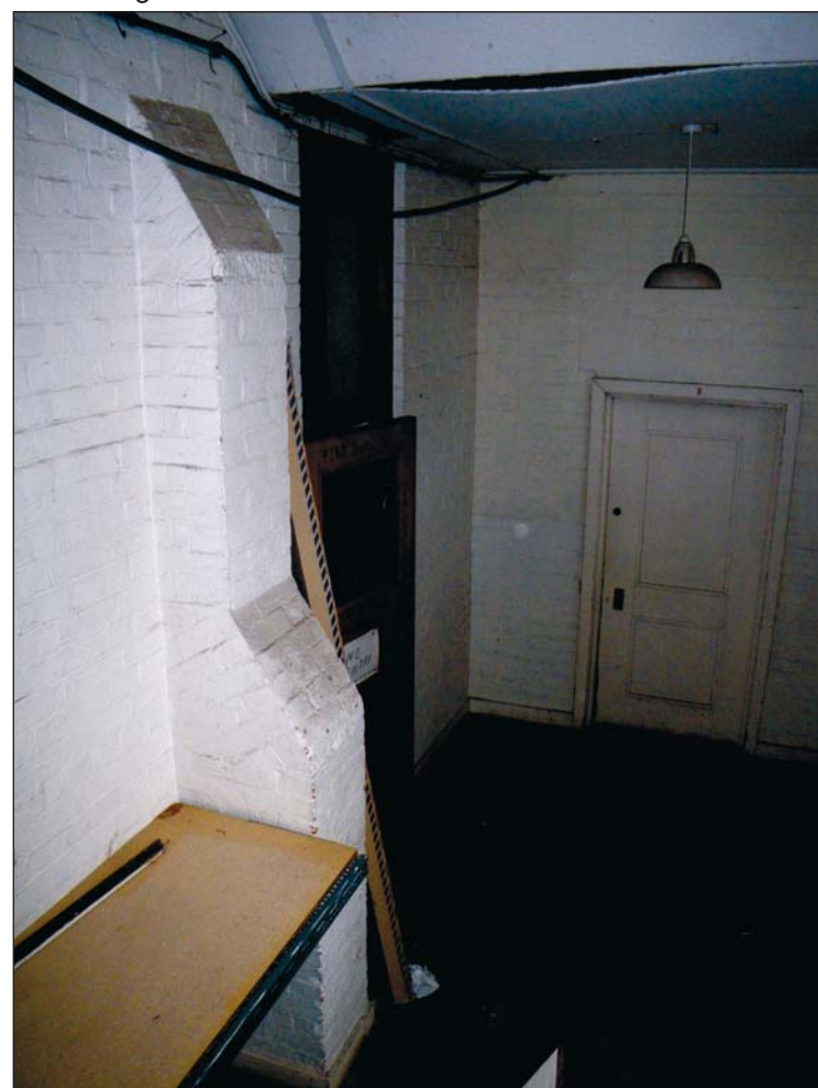
13 Two of the buttresses of the Period 1 building incorporated in the corridor on the south side of the Period 3 additions, looking east. The further one is in the wall and faint
