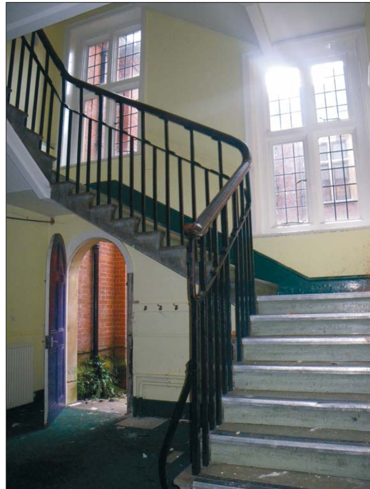
32 The Period 2 staircase ST5, looking south-west. The hand rail has been raised on extra ironwork for health and safety reasons
