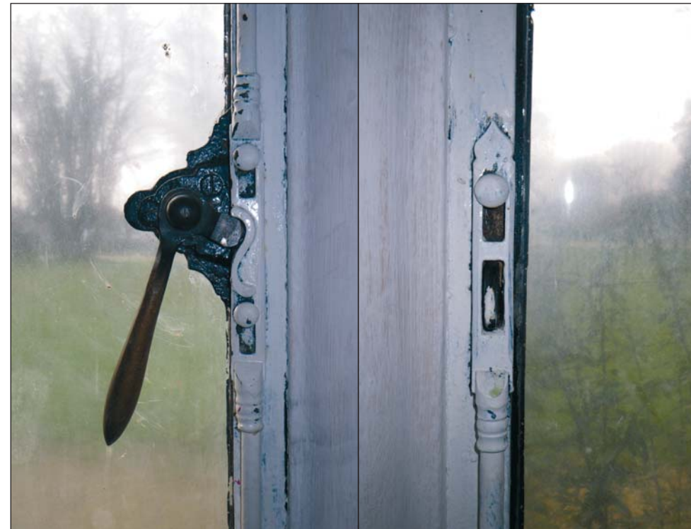
30 Period 1 window furniture in G11, typical of this phase in the building
