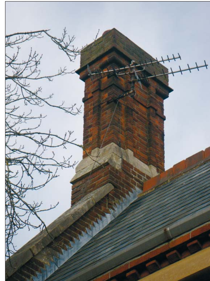
6 The chimney stack on the north end of the west wing, looking north-east
