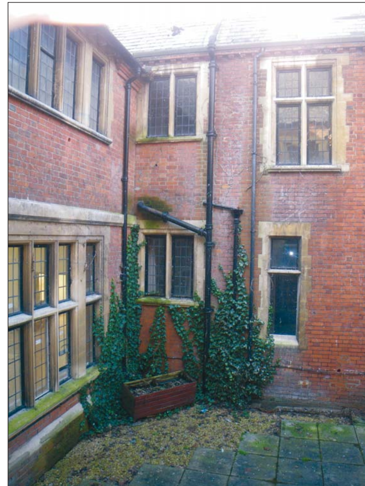
23 The south-west corner of the western courtyard, looking east The junction of the Period 2 building with the Period 1 is just right of the stench pipe. The top right window is a Period 2 insertion into the Period 1 wall
