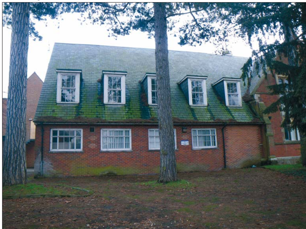
10 The north elevation of the Period 7 addition at the east side of the Period 1 hall, looking south
