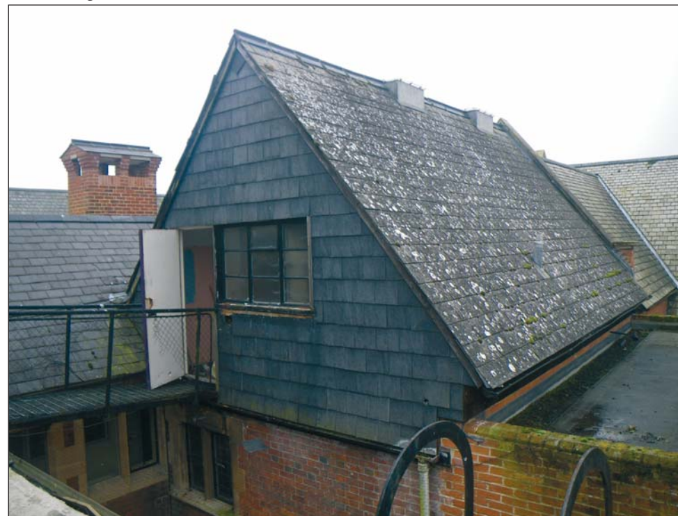
36 The added or rebuilt Period 3 roof over the Period 2 range north of ST5, looking south-east
