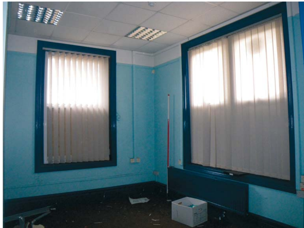
Fig. 17 The south-east ground-floor room in BD3 looking south-east, showing size of windows (and modern fittings) (Scale 2m)
