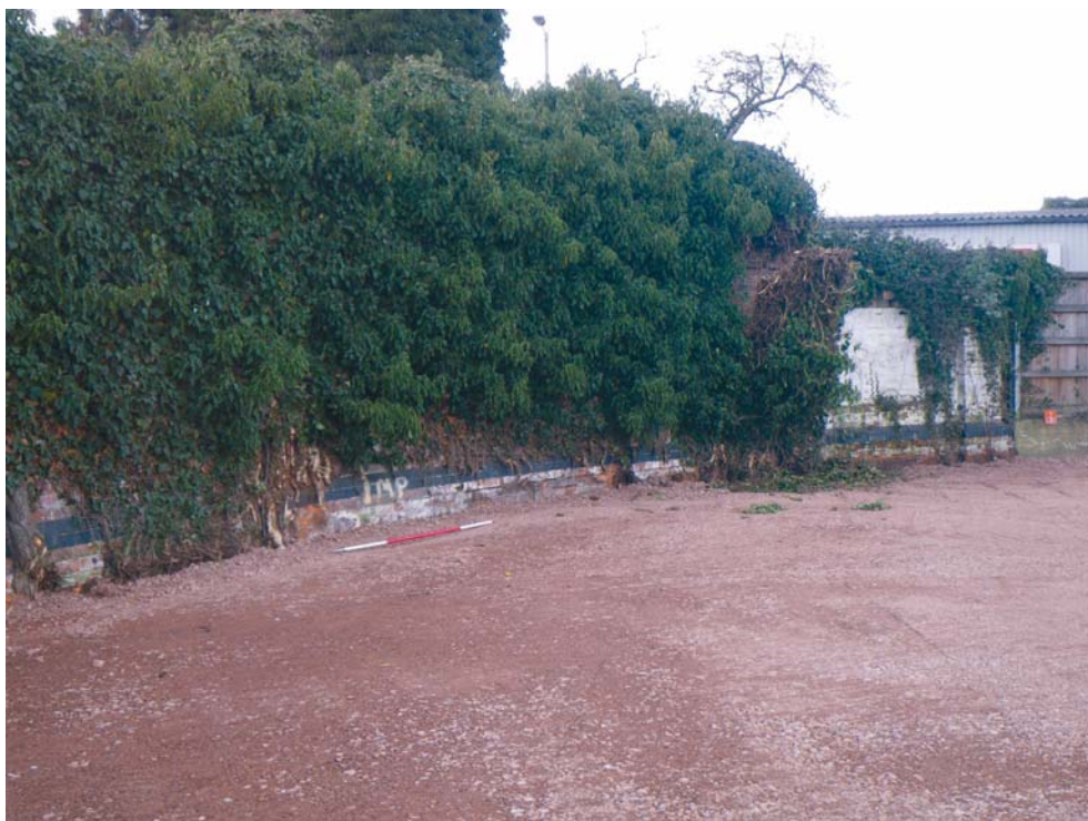
Fig. 30 The curved wall at the west end of the south part of the gasworks, looking west (Scale 2m)
