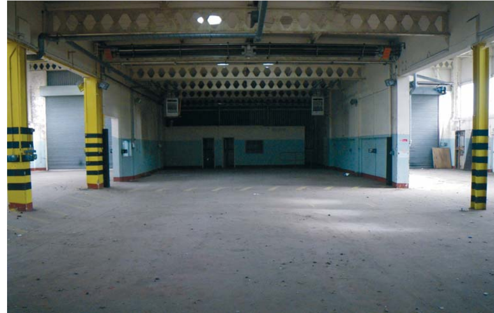
Fig. 44 The central "nave" of BD5, looking east, with offices at the far end and the heaters and ventilators slung from the ceiling
