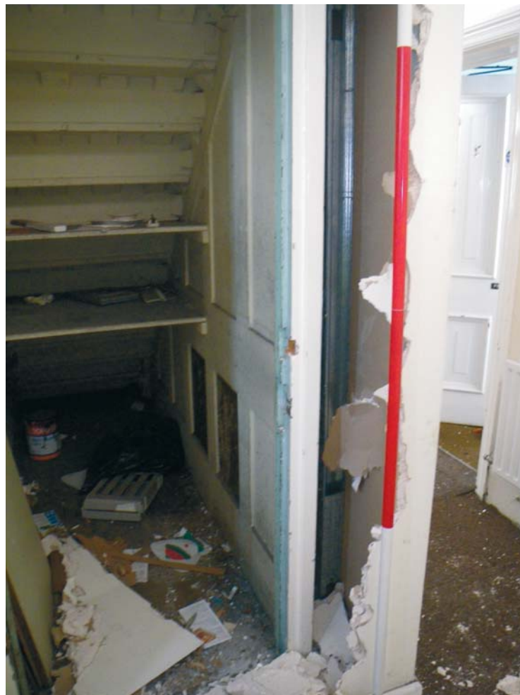
Fig. 20 The original under-stair cupboard and (rear of) panelling in BD3, with the remains of the recent fire enclosure, looking north-east (Scale in 0.5m divisions)
