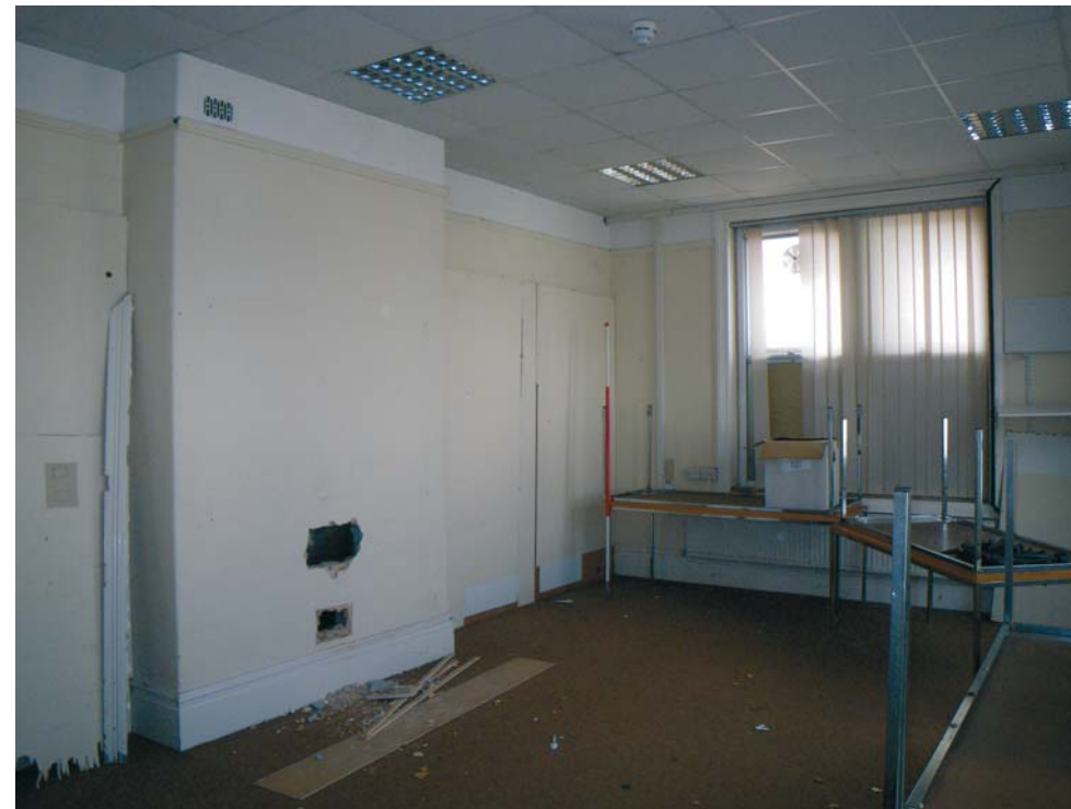
Fig. 18 The north-west room in BD3, looking south-west, showing false ceiling, blocked-in fireplaces and stud infill of the formerly-removed internal walls either side of the fireplace (Scale 2m)
