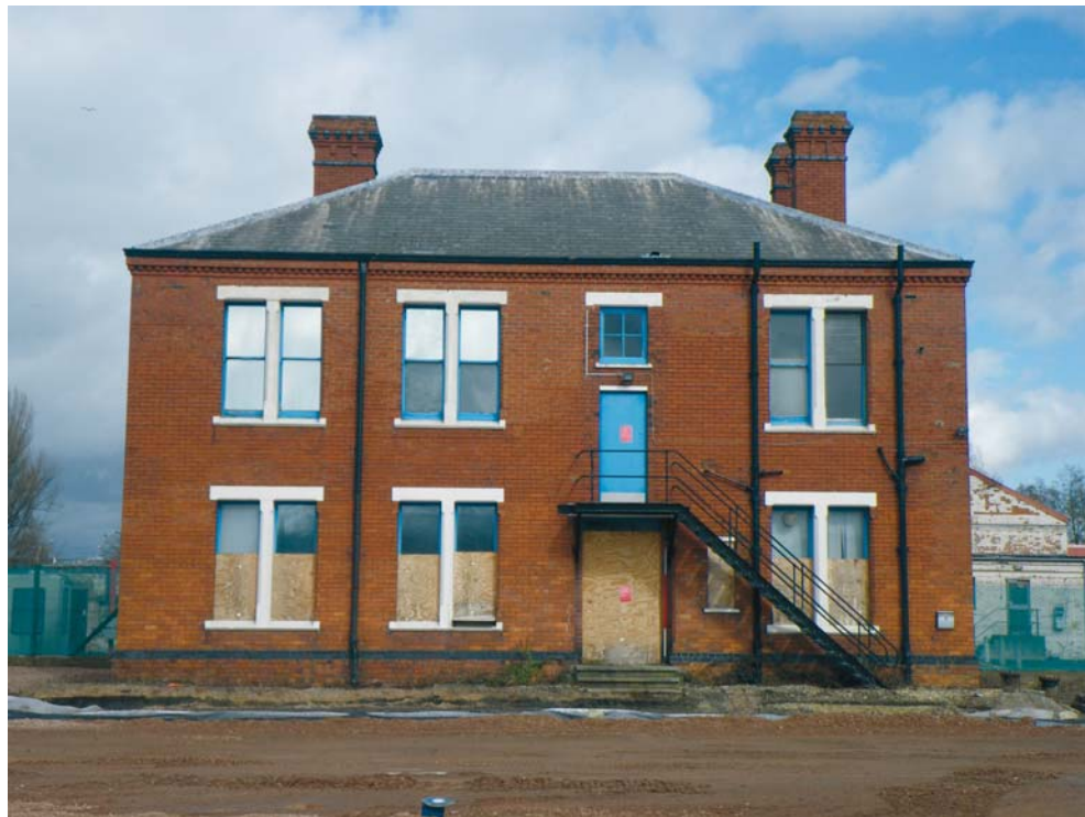
Fig. 24 The south elevation of BD3 showing the inserted fire escape door (and fire escape), converted window above it and the inserted window on the ground floor (Scale 2m)
