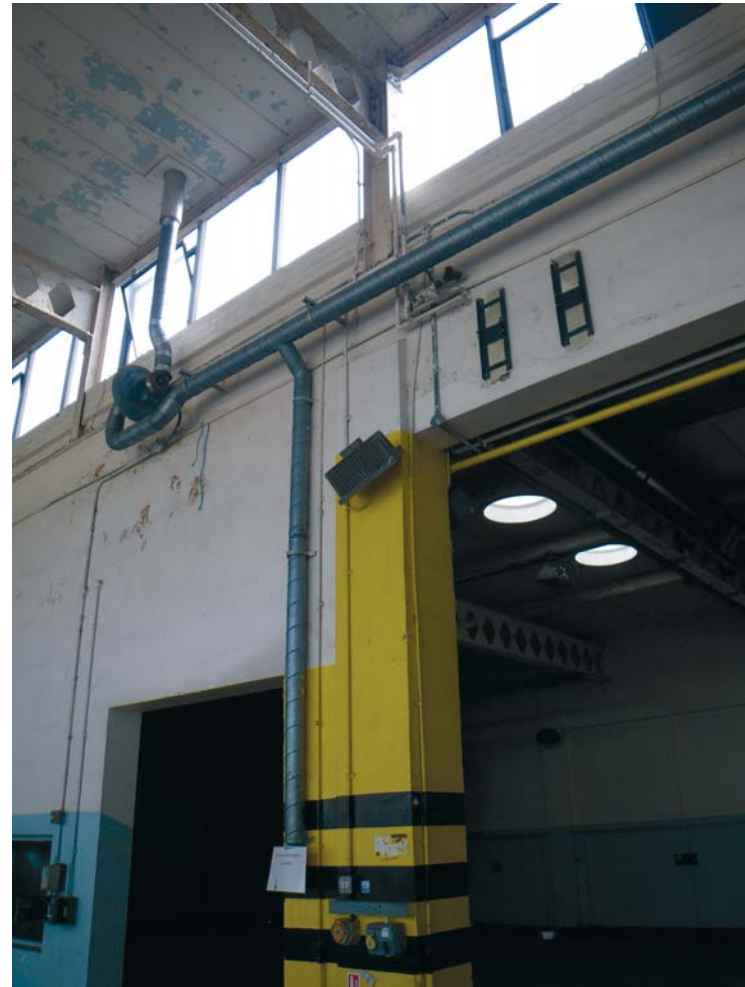
Fig. 43 The exhaust extraction system and one of the stations feeding into it in the north "aisle" of BD5
