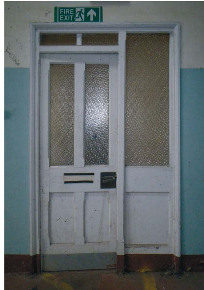
Fig. 40 The recycled door and partition at the east end of the corridor in the north-west corner block of BD5, seen from the "transept", looking west
