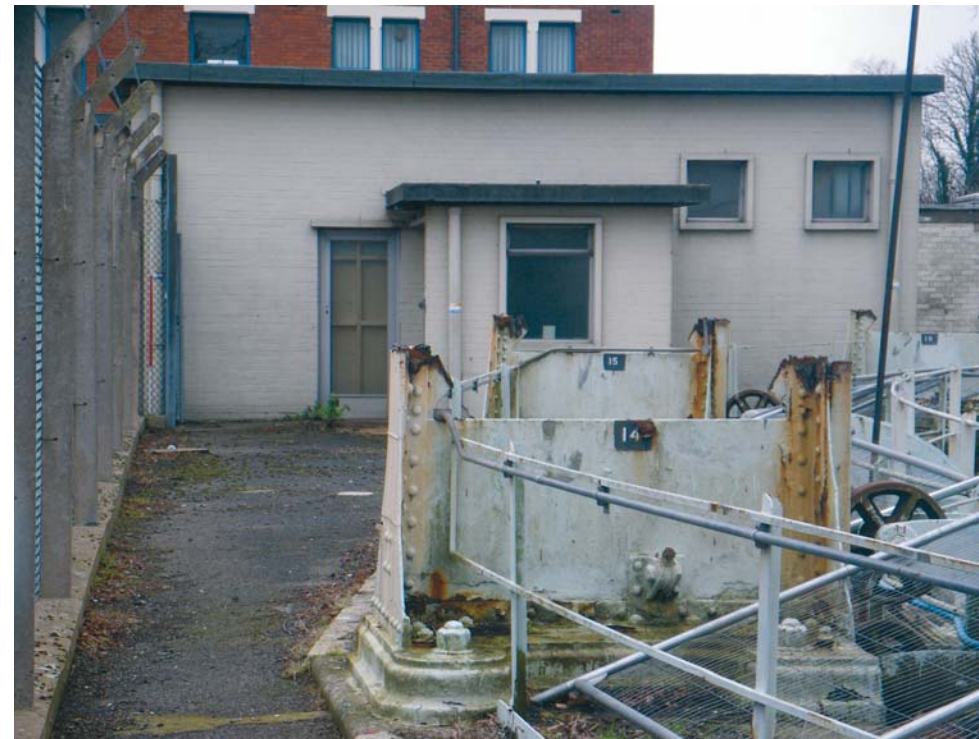
Fig. 14 The north elevation of BD2, with the 1901 gasometer stanchion stumps visible in foreground (Scale 2m)
