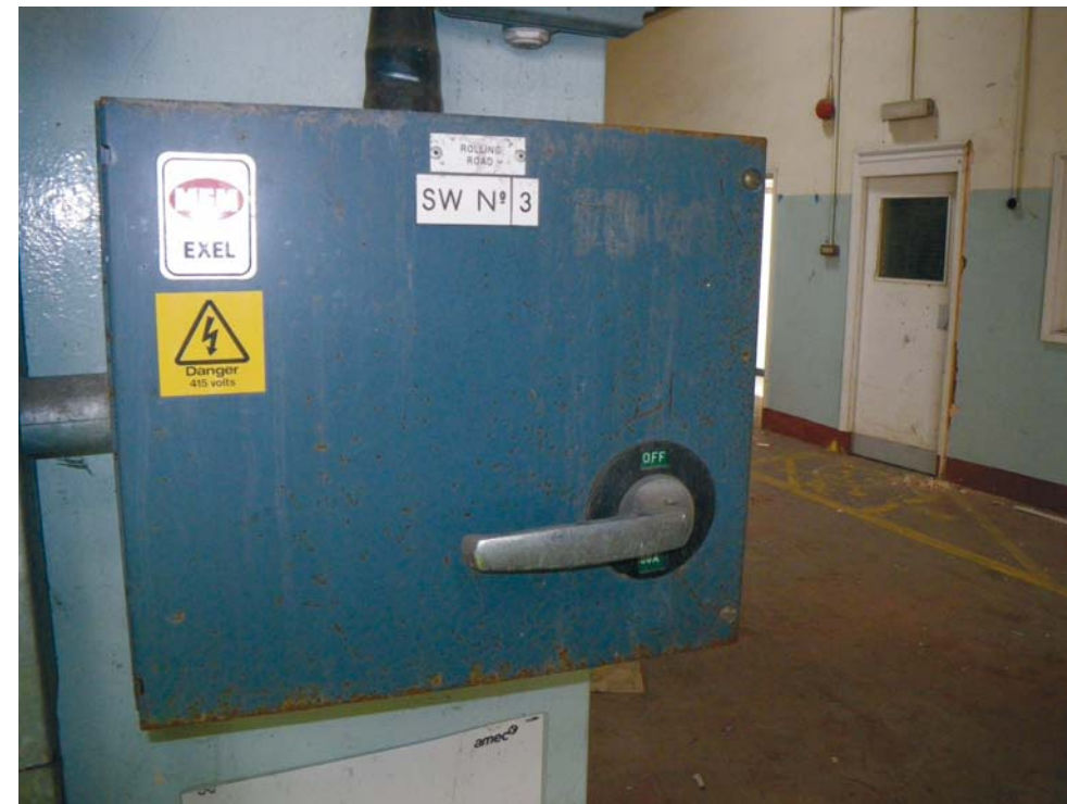
Fig. 42 The control box for the rolling road in BD5, on the wall nearby
