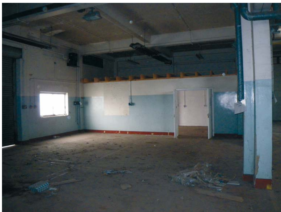
Fig. 37 The western central room of BD5 and the office inserted into the northern side of it, looking north-east
