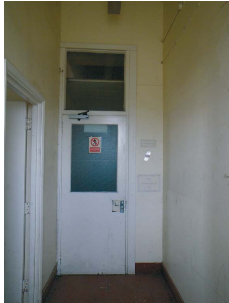
Fig. 39 The door from the (full height) entrance lobby in BD5 into the corridor in the north-western corner block, looking east. Note the false ceiling behind the transom light
