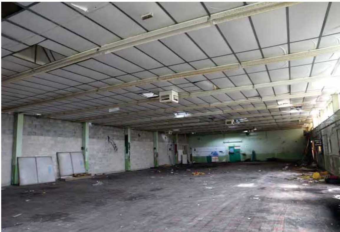
Plate 77: Design Office –interior view of the western half. Shows the cased columns and false ceiling hiding the roof structure
