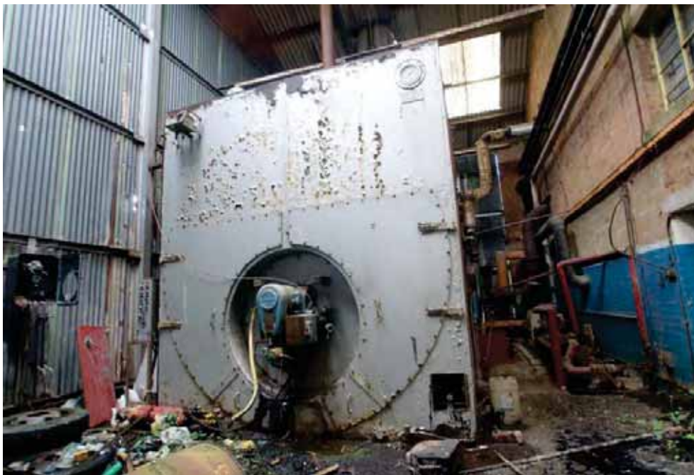
Plate 46: Interior of the new boiler house showing the boiler, July 2015
