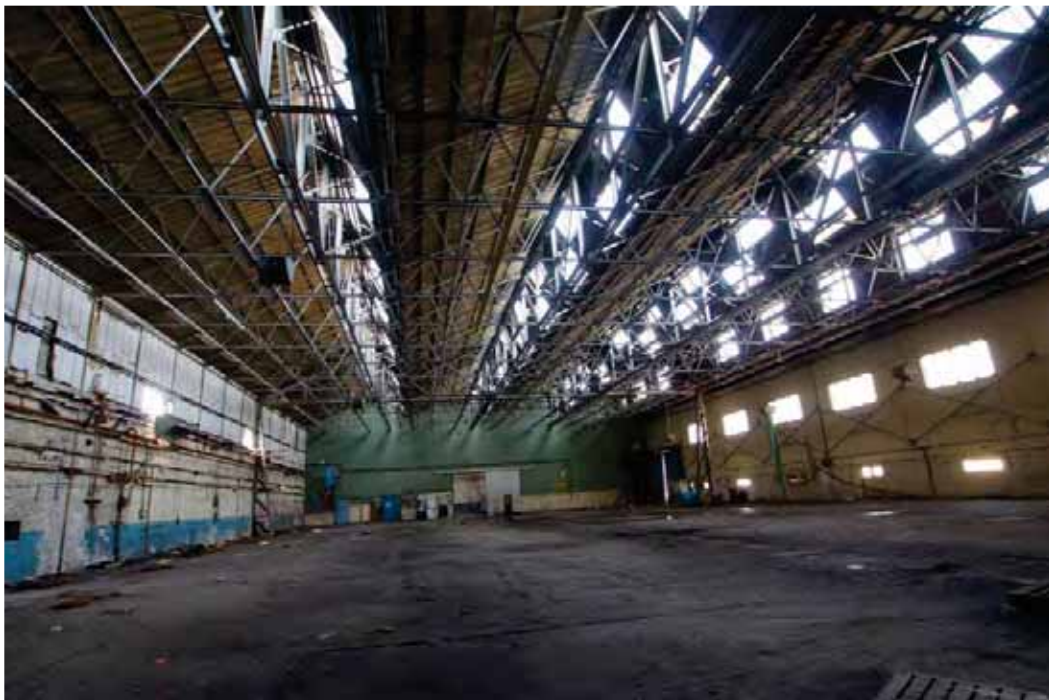
Plate 33: Flight Shed No.1 – interior view looking to towards the fire break and 'A' frame
