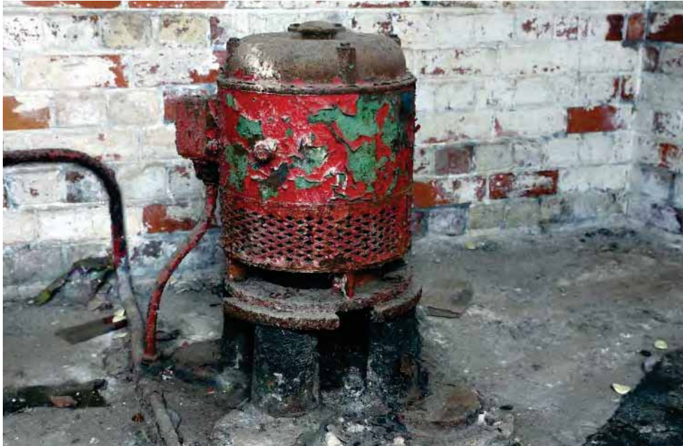
Plate 26: Motor inside pump house, building 148 July 2015
