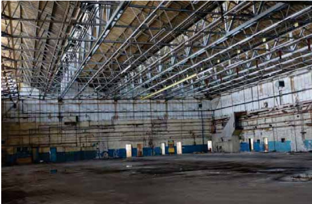
Plate 34: Flight Shed No.1 – interior looking towards the smaller half of the shed at the west end wall
