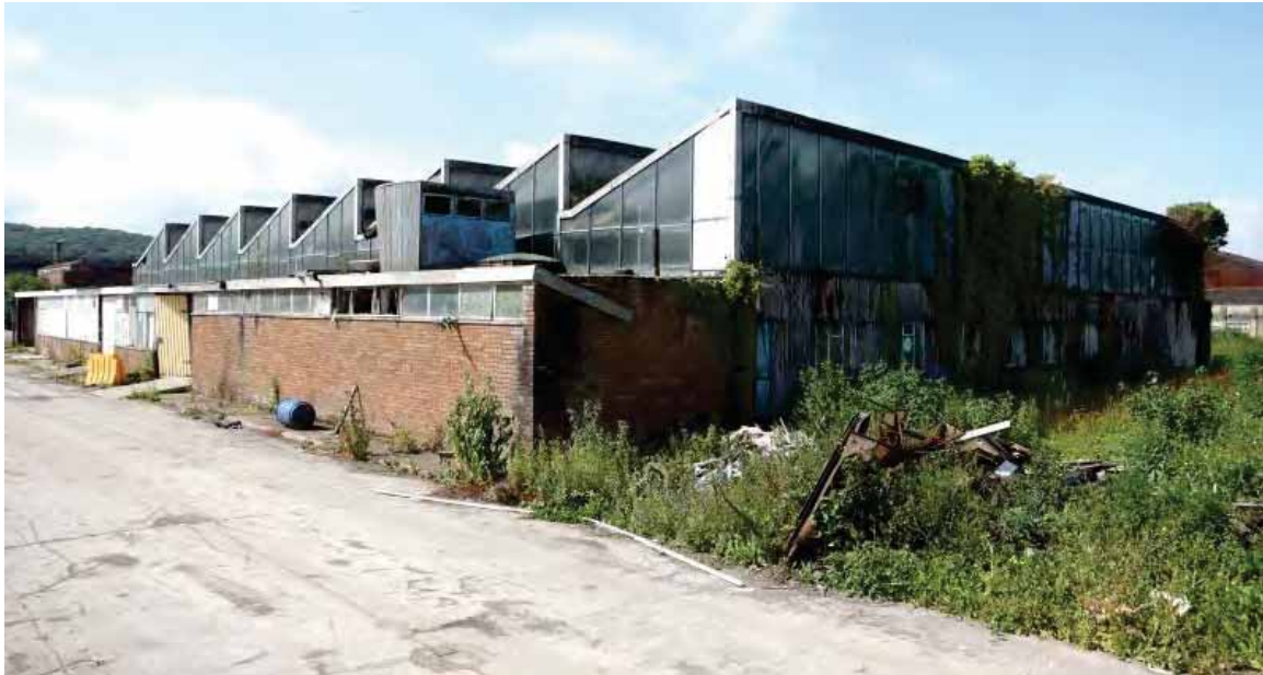
Plate 76: Design Office – view looking south-west. The northern gable end elevation still shows signs of its original wall cladding
