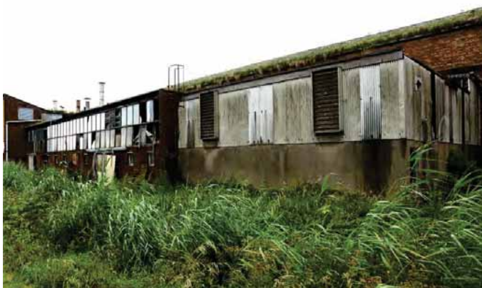
Plate 60: Shop 7 – external view of the treatment room with the plant room on right
