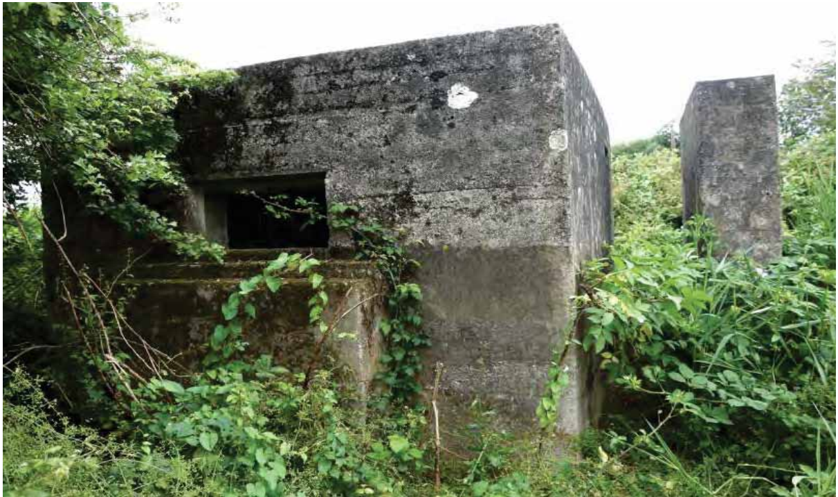
Plate 13: Type FW3/26 Pillbox on Defence Site No.4, (Bldg.104) - Note the thickened section below the loophole facing the airfield (July 2015)
