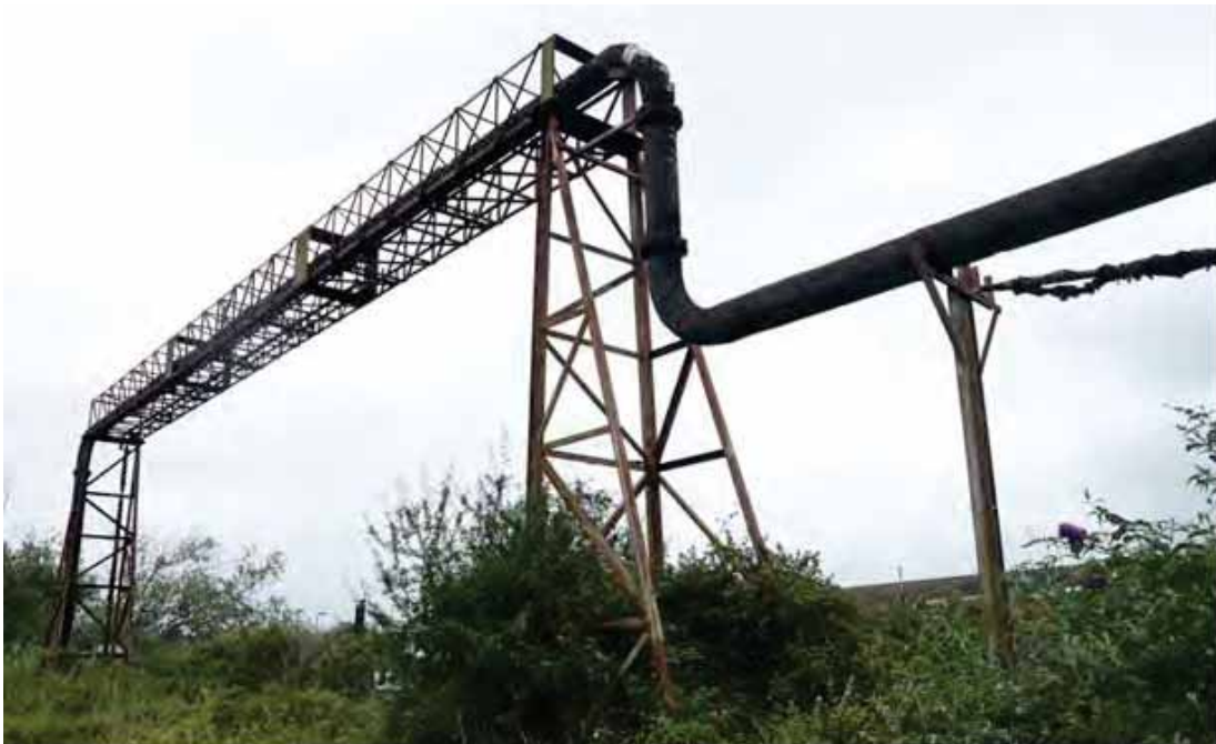
Plate 1: Heating pipe gantry where it rises over an access road over the Cross Rhyne
