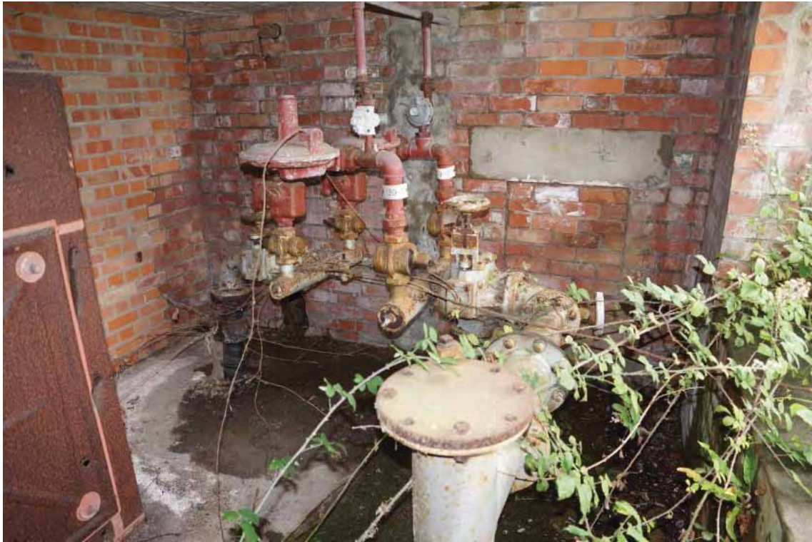
Plate 84: Plant equipment in Bldg 147
