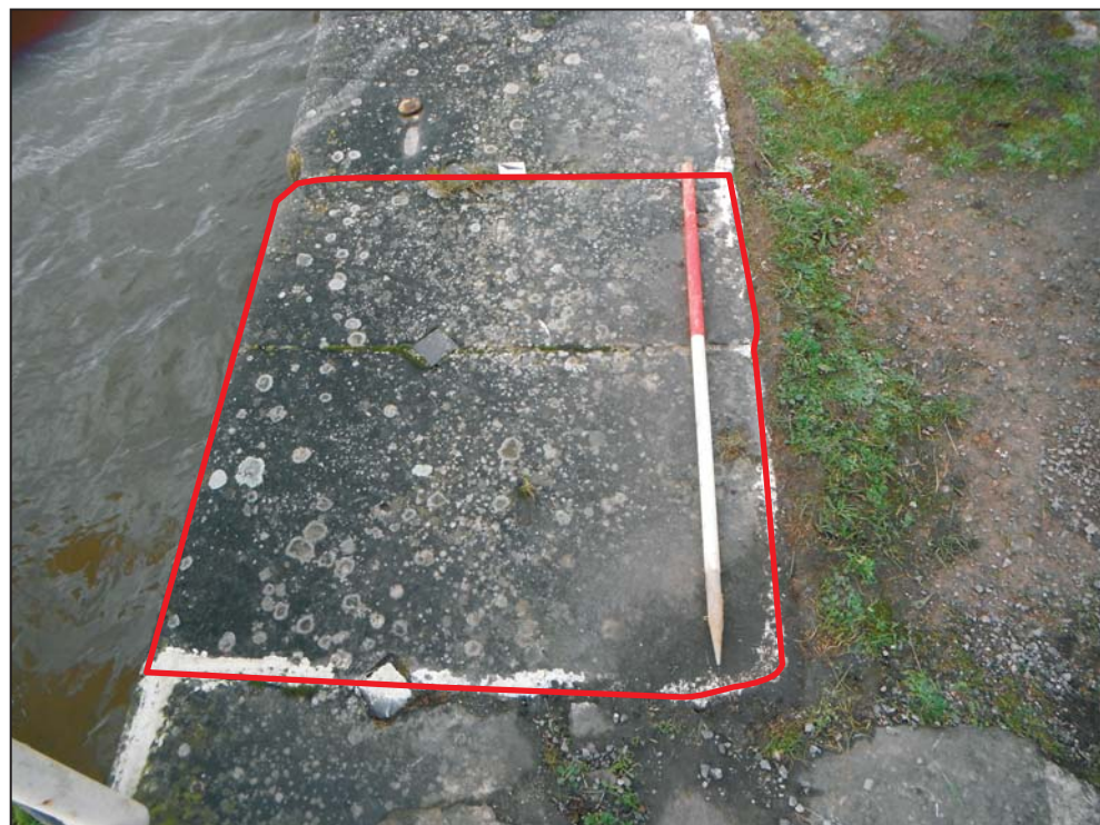
Stones affected by works (highlighted), looking west (1m scale)
