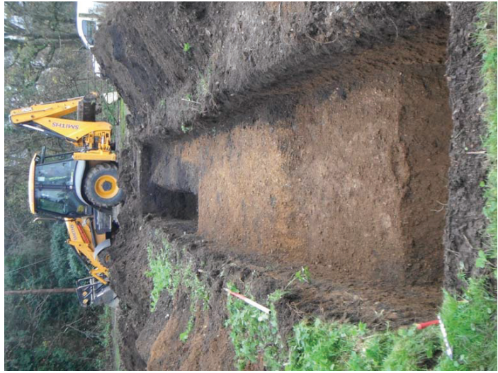
Trench 2 looking south-east; undated pit [213] in foreground, modern pit [209] to rear. (1m scale)
