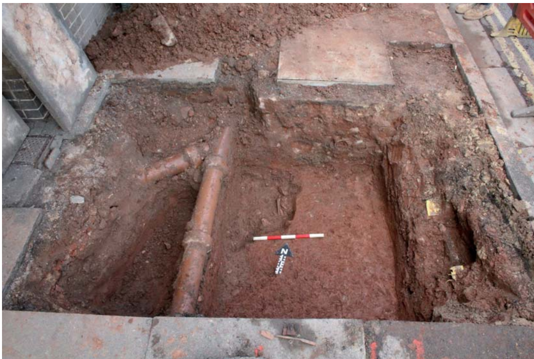
Excavated trench showing grave cut 106 with heavily disturbed burial 105. Newly installed PCP119 cabinet ducting manhole is visible to the top of the photograph. Also showing ceramic storm drains to the left and the electric cable to the right. Looking north (0.5m scale)
