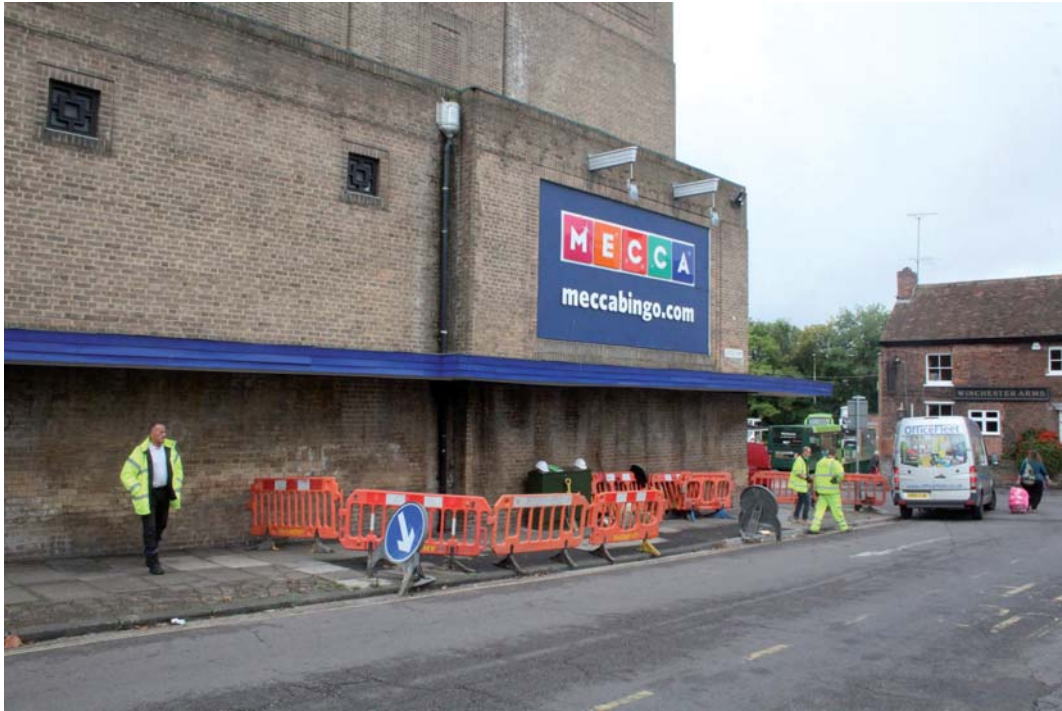
General view of the trench, showing location of the installed green new PCP119 cabinet against the Mecca Bingo building, looking north-west
