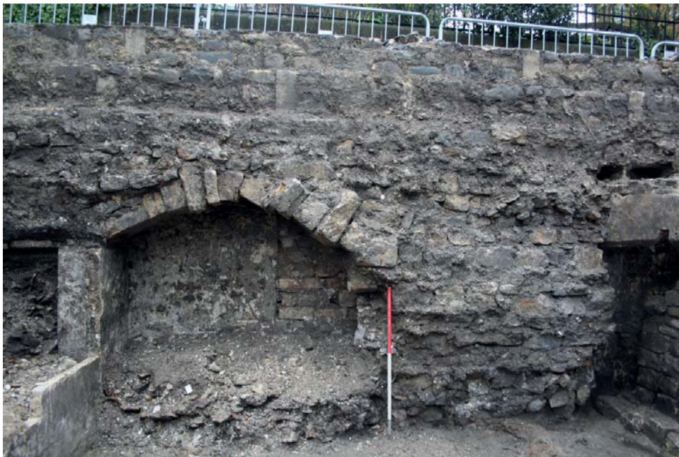
No. 9 Bridewell Lane, showing the 'relieving arch' in the later wall with the early wall and blocked doorway leading below the lane, looking east (scale 1m).
