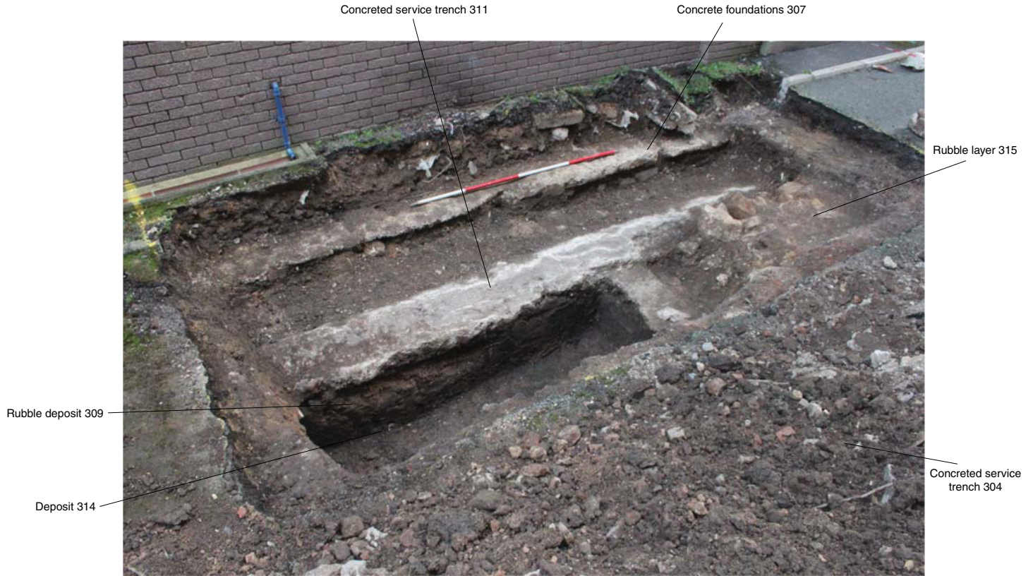
Trench 3, looking south-east, showing foundations and services associated with C wing (2m scale)
