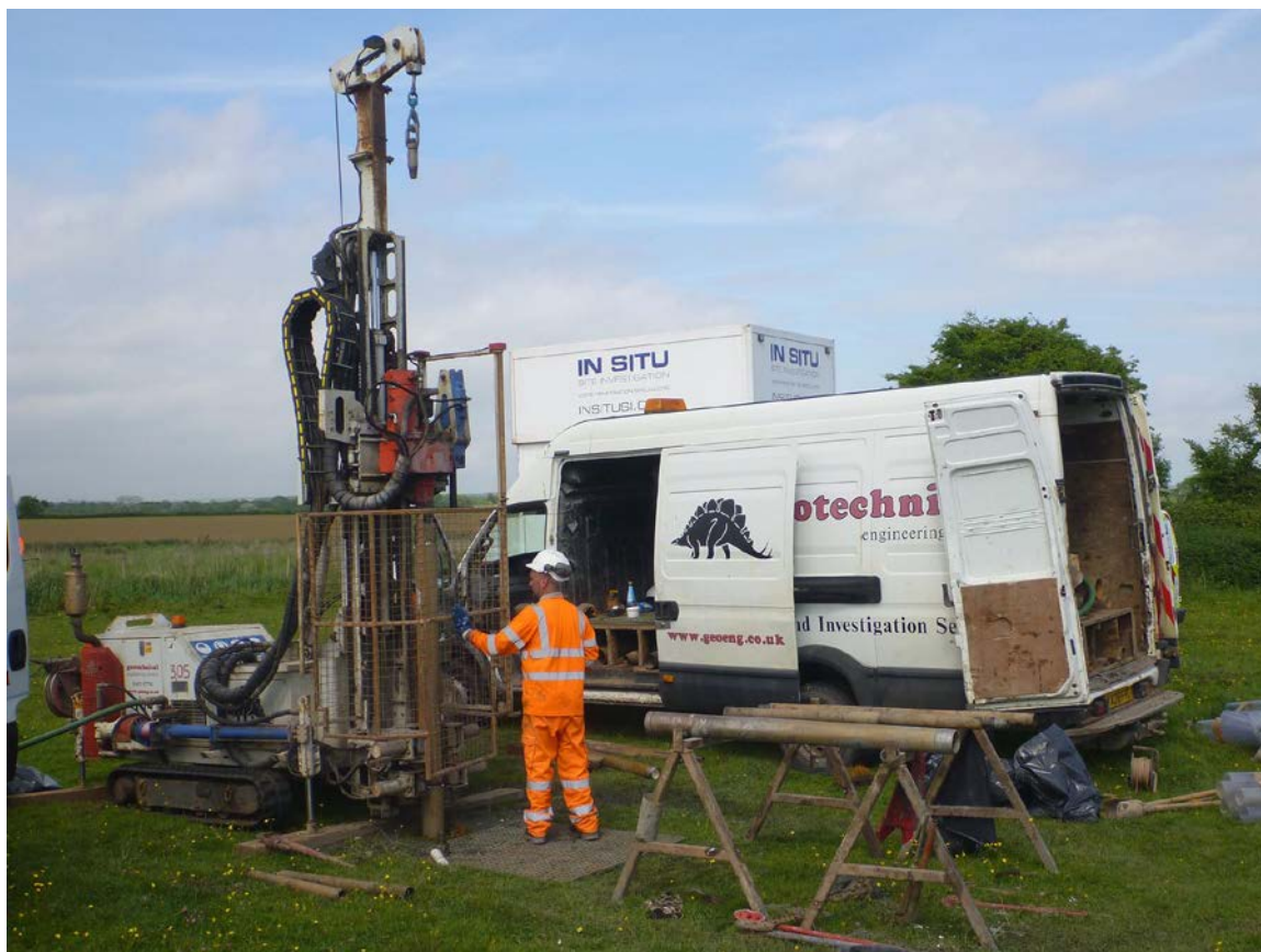
Figure 2. Technicians from GE employing a Pioneer 2 rig to advance ARCA BH1. Casing is being inserted into the borehole to prevent collapse of the walls, while core chambers are lying on the trestles
