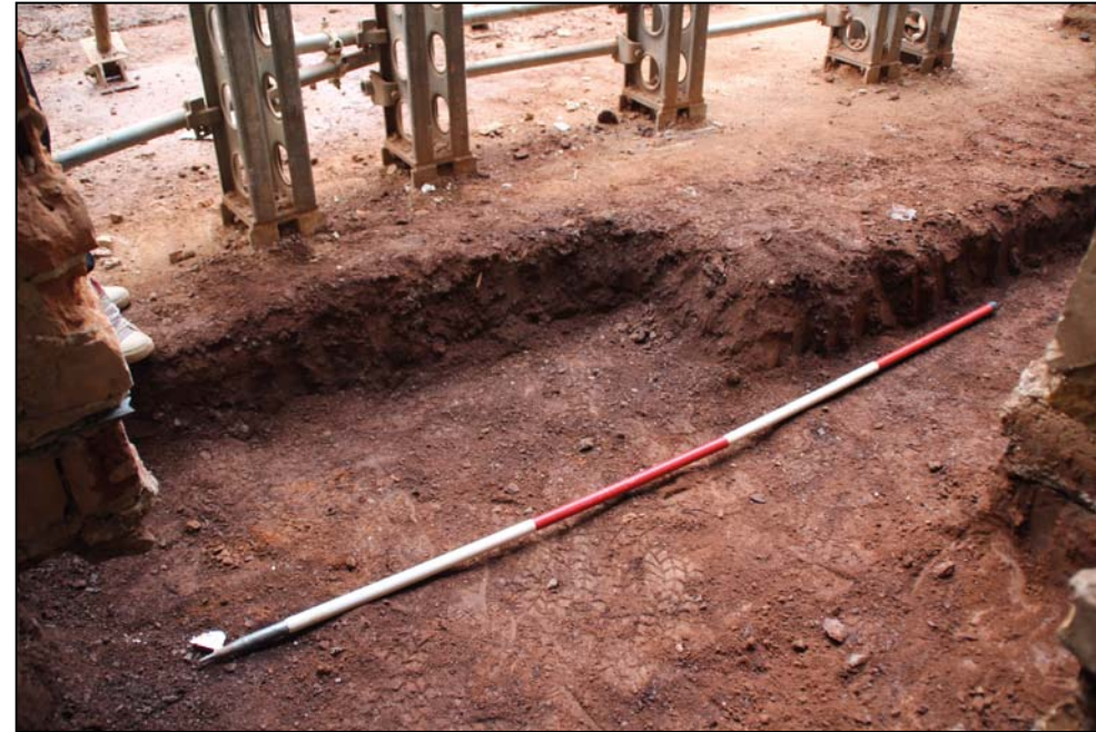
Figure 43: Excavations at the rear of the west wing, looking north-east. The level supporting the props has been reduced by 300mm and the deeper area by another 250-300mm, exposing only degraded sandstone natural (scale 2m)
