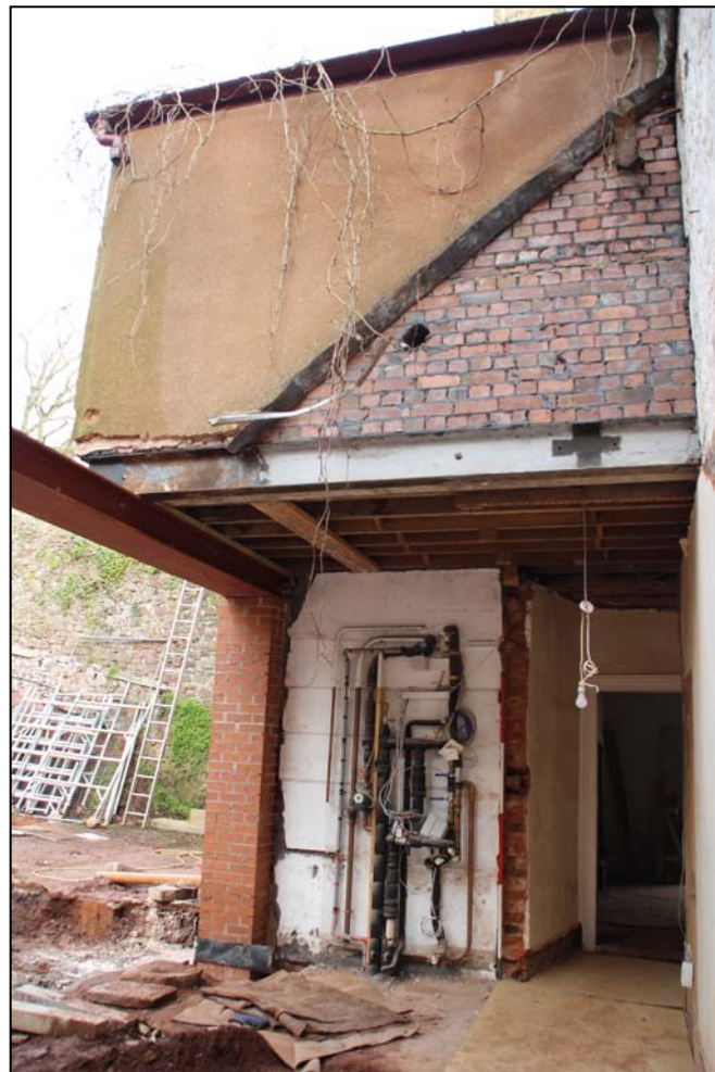
Figure 18: The first floor bathroom after demolition of the eastern utility room and rear corridor and the insertion of the modern steel and brickwork to support the old steel and brick, looking east, (scale 2m)
