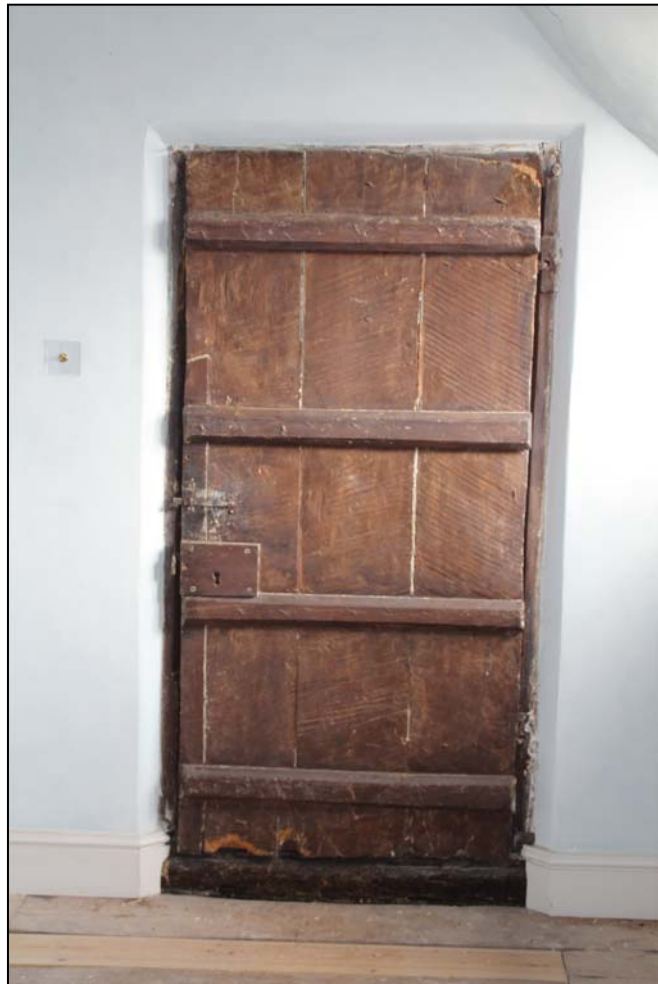
Figure 36: The door and doorframe between Bedrooms 7 and 8
