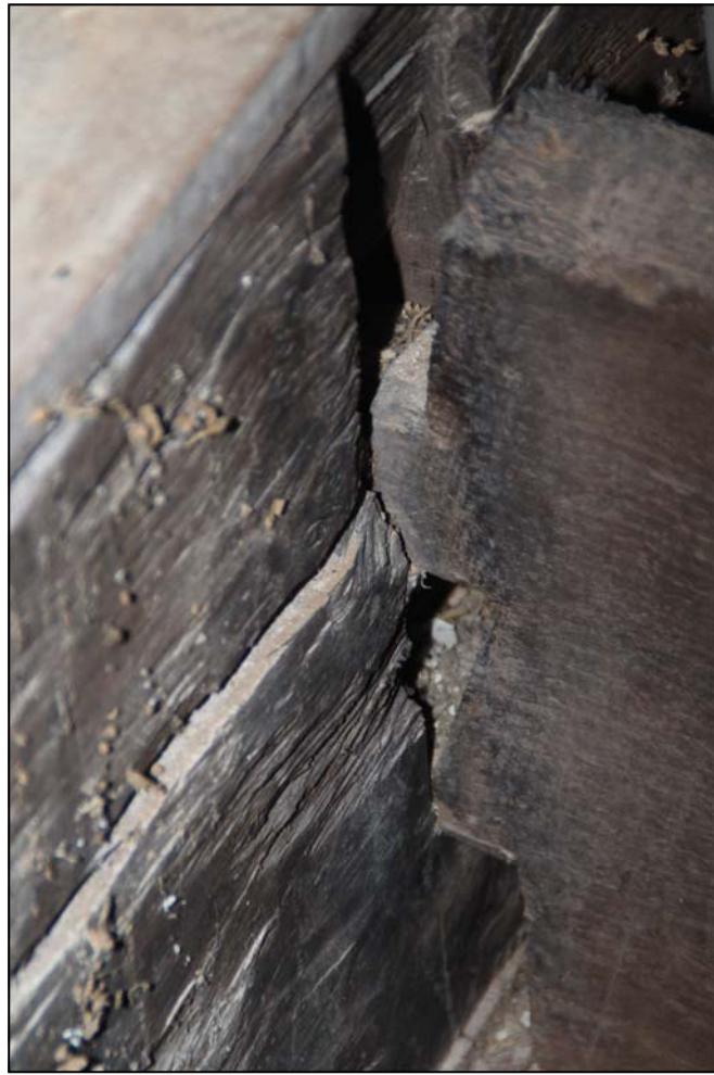
Figure 34: The mortise and tenon joint of the joists and beam in Bedroom 8
