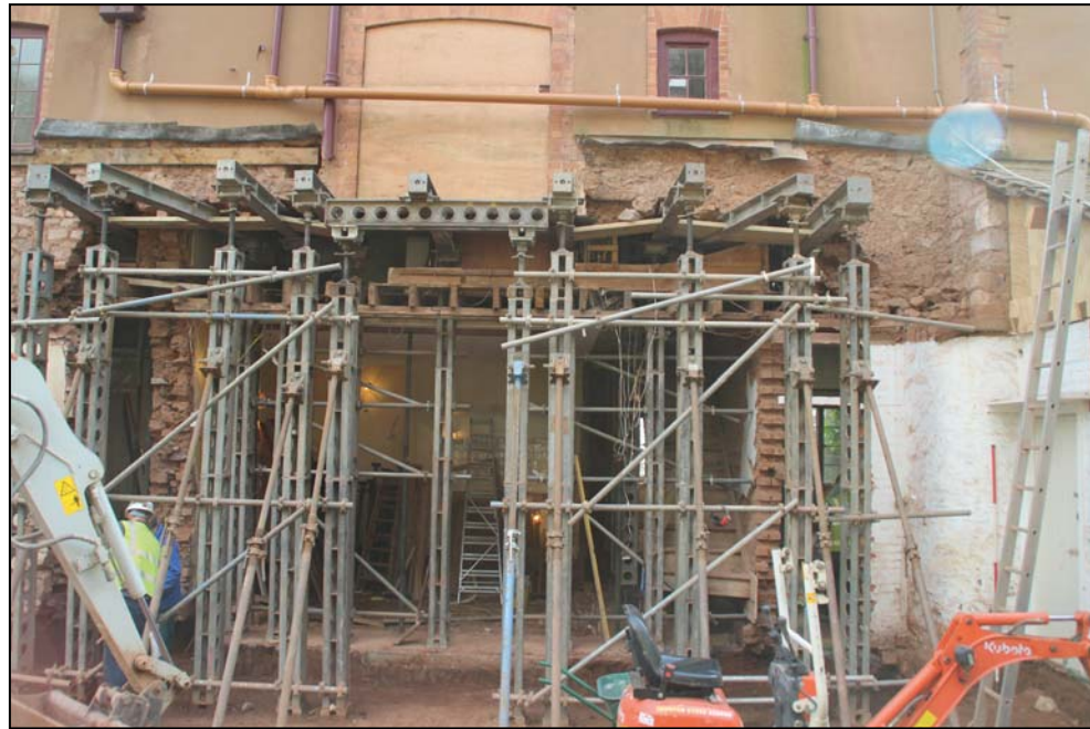
Figure 14: The rear wall of the west wing after demolition of the rear ranges and the lower part of the wall. Note stack quoins on right (scale 2m)
