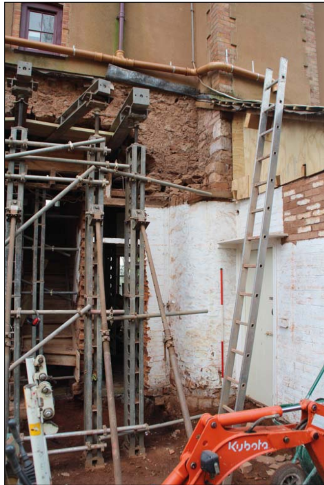
Figure 16: The stack at the north end of the west wing, continuous with the older masonry of the north wall, to south-west from within the demolished western utility room.
