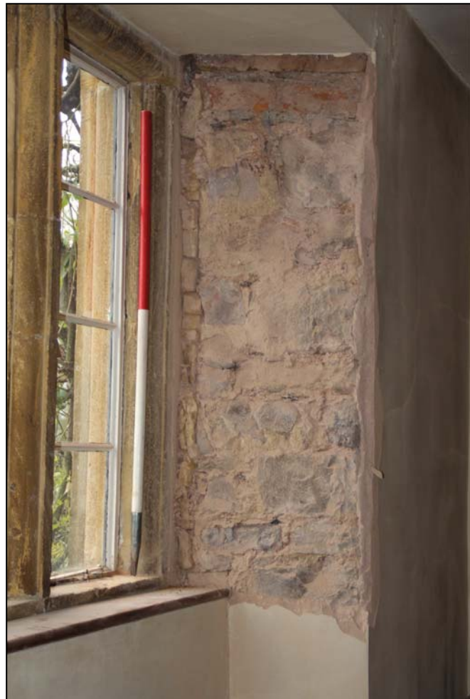
Figure 24: The stripped west splay of the south window in Bedroom 1, showing brick repair and modern plaster (scale 1m)
