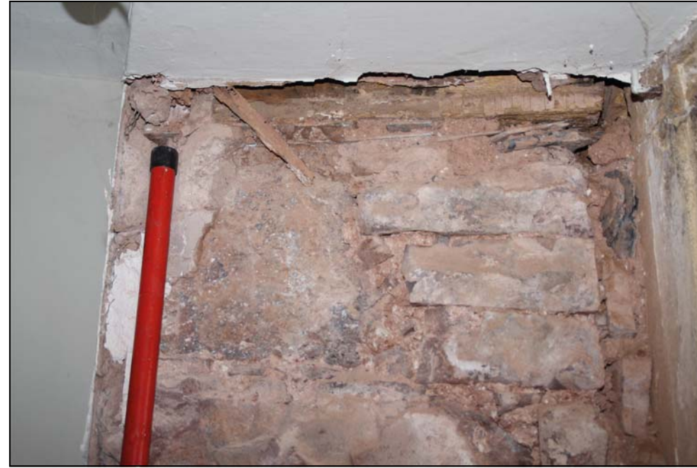
Figure 7: Timber pad at the top of the reveals in the mullioned windows (here in the Sitting Room (hall) eastern window, looking east)
