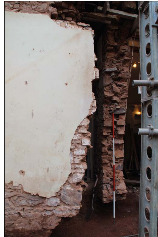
Figure 17: Cross-section of the west wall of the central range, no footings and relatively regular construction, looking south-south-west, 19th-century wall in front (scale 2m). The concrete scraps are the remains of the silver safe
