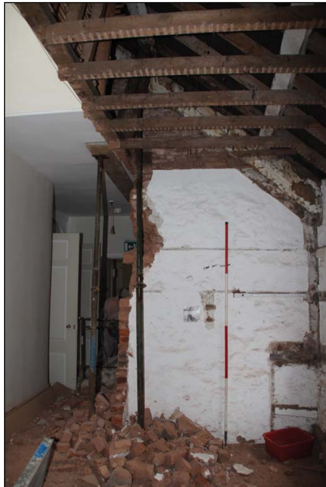
Figure 20: The eastern utility room looking west after the demolition of the brick wall forming the rear corridor: inserted 1930 ceiling joists below the 19th-century roof timbers
