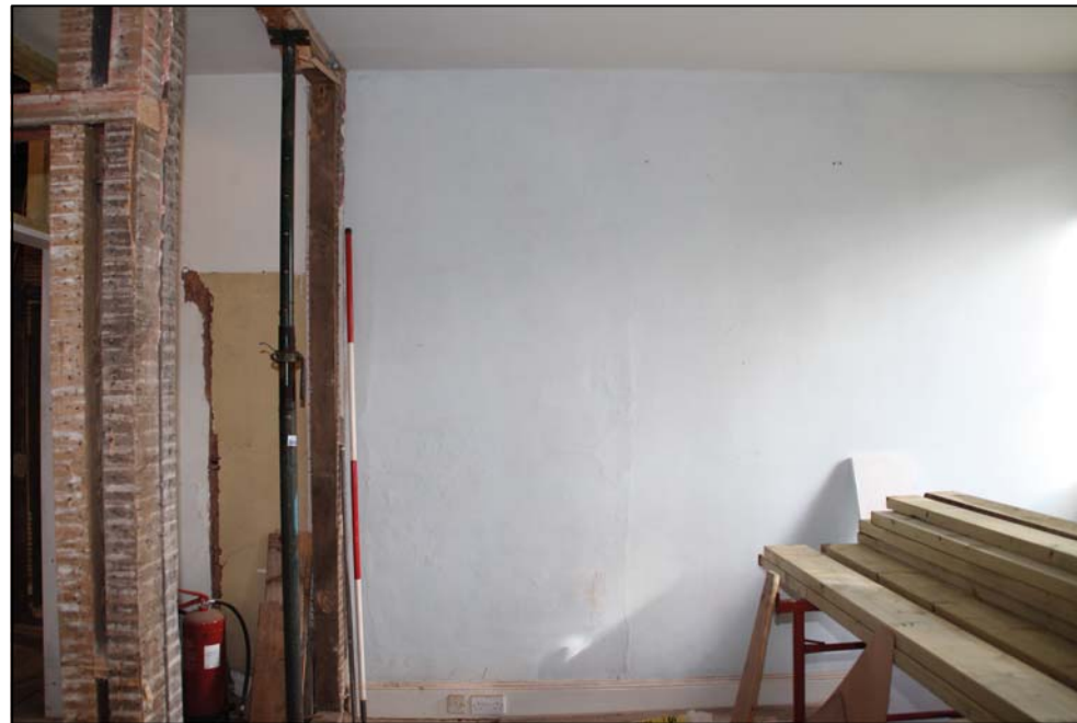
Figure 29: The blocked doorway in the wall between Bedrooms 4 and 5, looking east (scale 2m)
