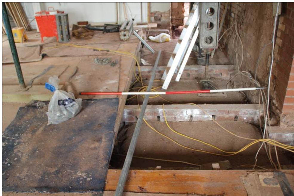
Figure 12: The possible barrel-vault extrados under the rear part of the Games Room, looking north (scale in 0.5m divisions)
