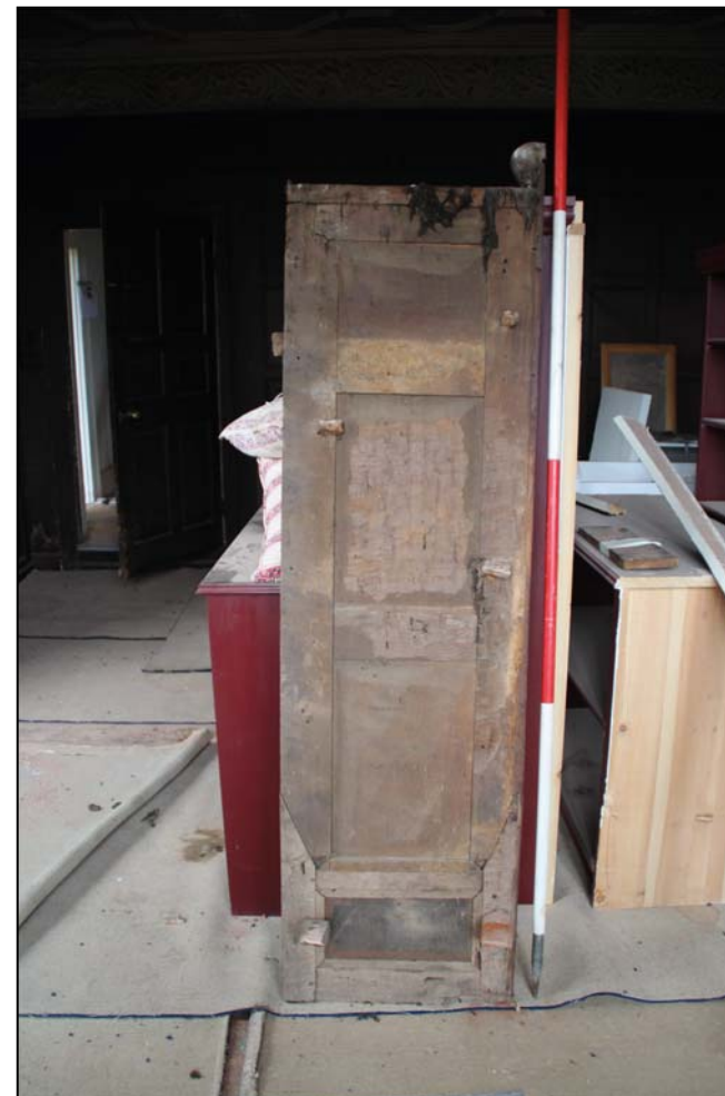
Figure 9: The rear face of the panel removed from the reveal in the Drawing Room; note repair (scale in 0.5m divisions)
