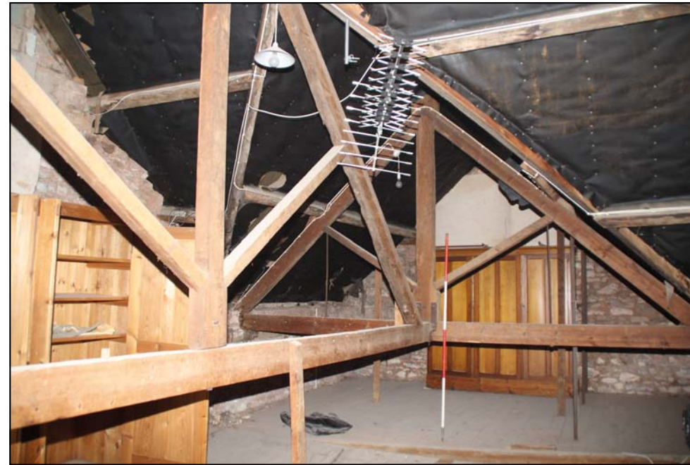
Figure 39: The western truss of the main roof supported by the east/west truss of the western rear roof, looking north-north-west (scale 2m)
