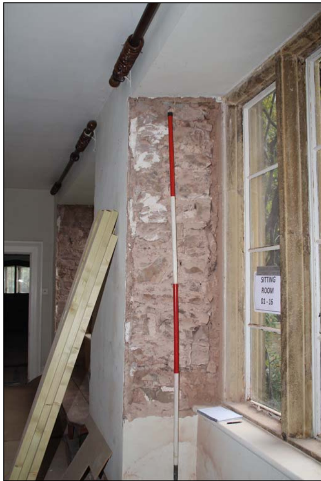
Figure 6: The reveals of the windows in the Sitting Room (hall) stripped plaster, looking east (scale in 0.5m divisions)
