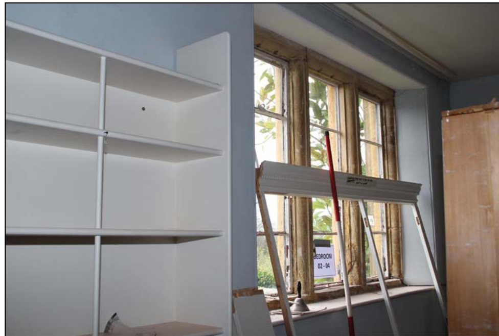
Figure 25: The western window in the south side of Bedroom 5, showing probably re-used mullions, cills and lintels with filled bar-settings visible in the lintels (scale in 0.5m divisions)
