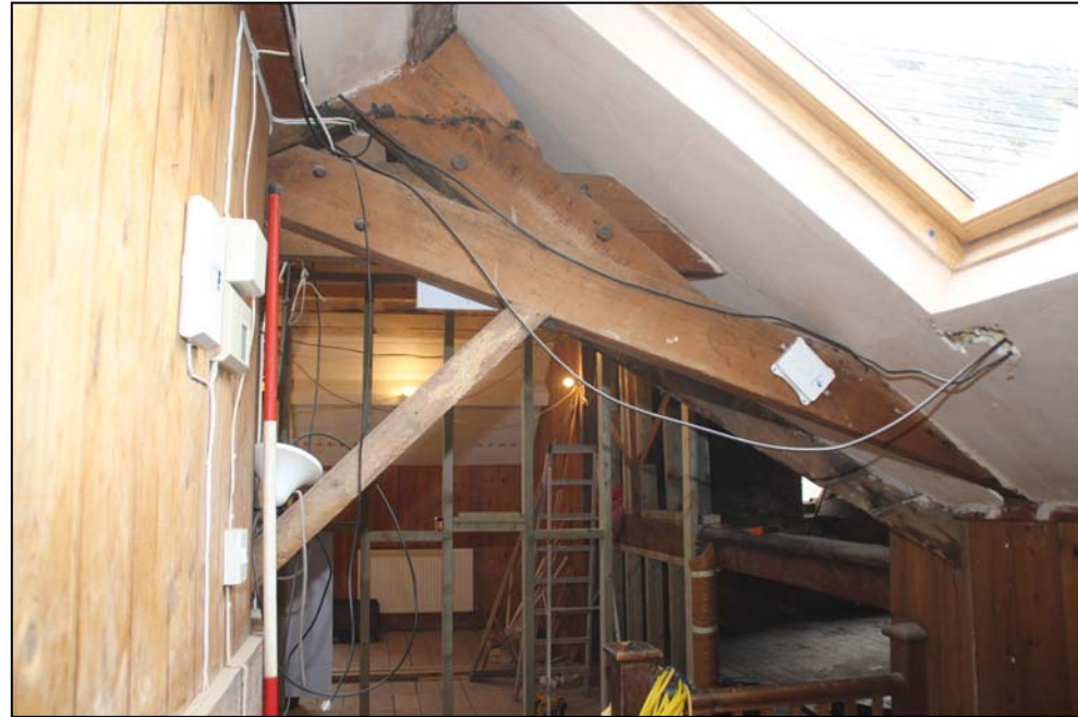
Figure 42: Timbers inserted in 1930 to replace and support removed and truncated timbers, from the top of the back stairs, looking south (scale in 0.5m divisions)
