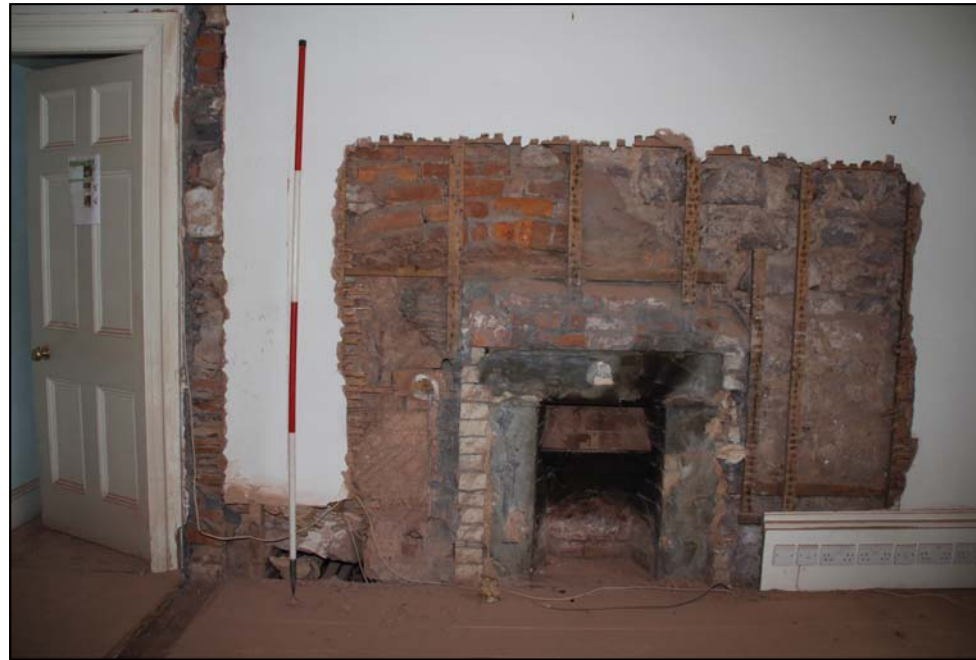
Figure 23: The blocked fireplace in the north wall of the office after removal of lath and plaster covering (scale 2m)
