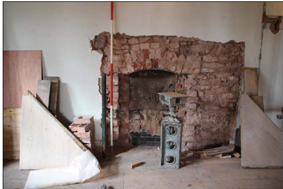
Figure 32: The fireplace recess in the north wall of Bedroom 6 (scale in 0.5m divisions)
