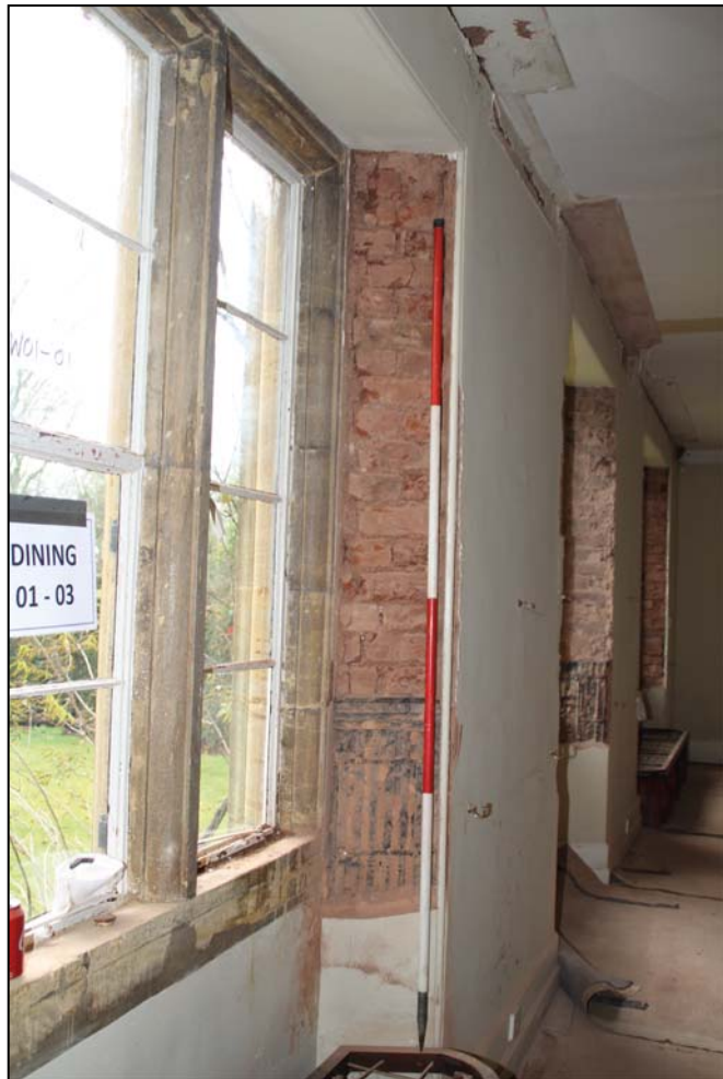
Figure 10: The brick reveals of the Games Room windows and the probably re-used windows, looking W (scale 2m)
