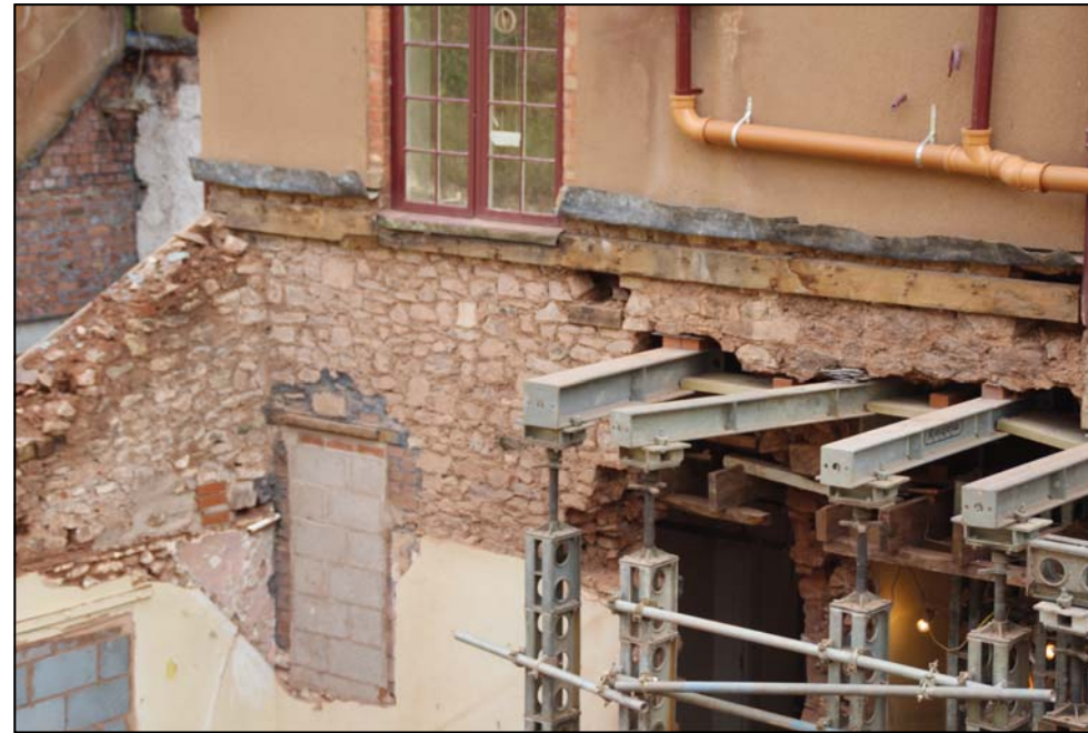
Figure 15: The junction of the older masonry at the rear of the west wing (over the needles) with the rubble walling of the 19th-century rear range (bathroom and central larder), looking south-east
