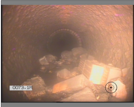
Photo: 4_18A, 00:06:53 73.1m, Settled deposits, coarse, 40% cross-sectional area loss
