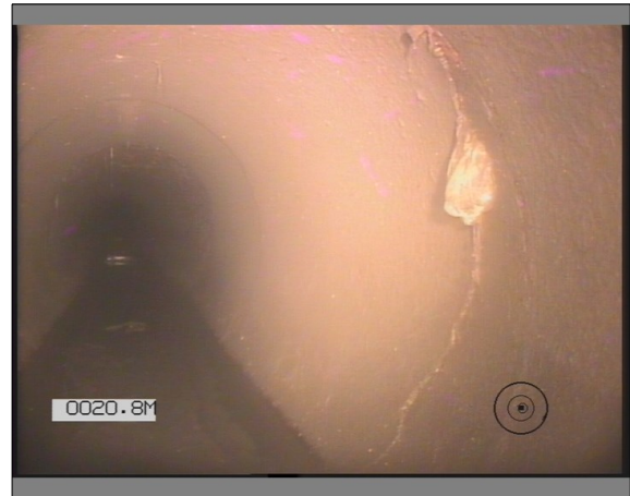
Photo: 4_5A, 00:01:47 20.8m, Fracture, circumferential at joint, from 2 to 5 o'clock
