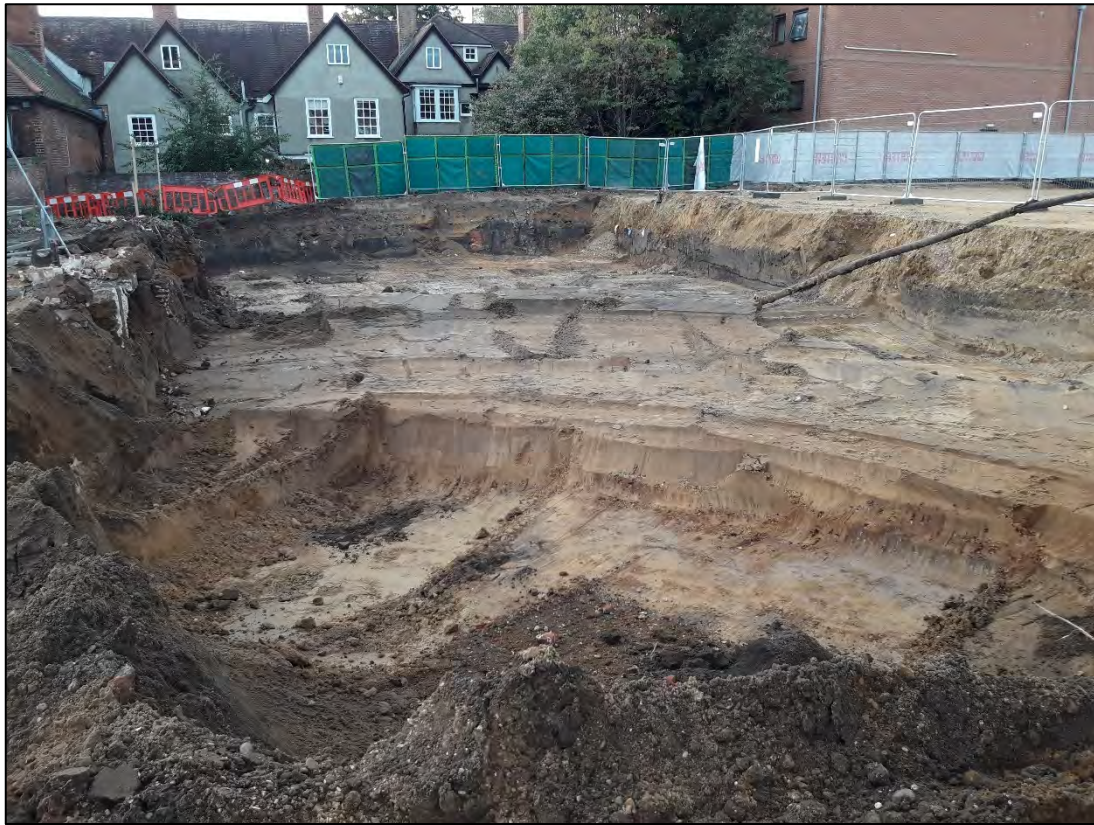
Plate 28. Subsoil layer 0004 in the northwest corner of the site, during stripping. Looking west
