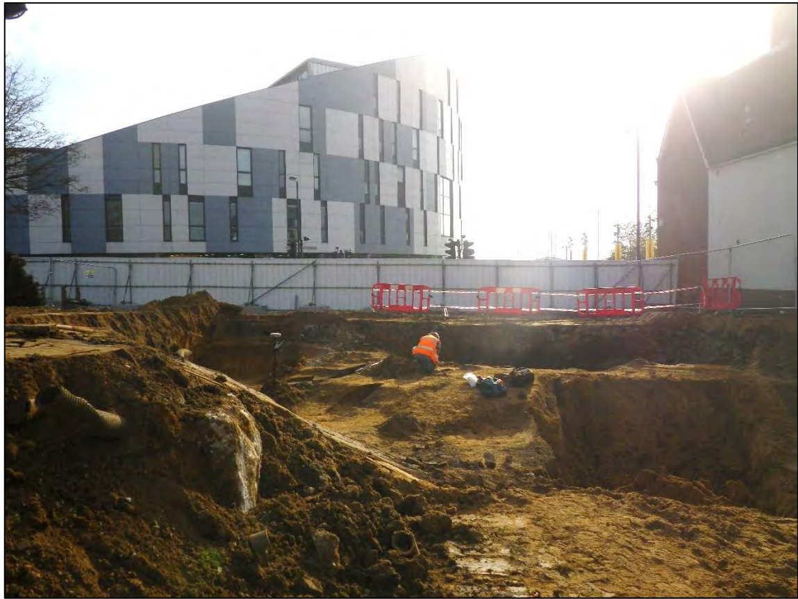
Plate 4. The southwest corner of site, showing the results of contractors' machine strip. Looking south
