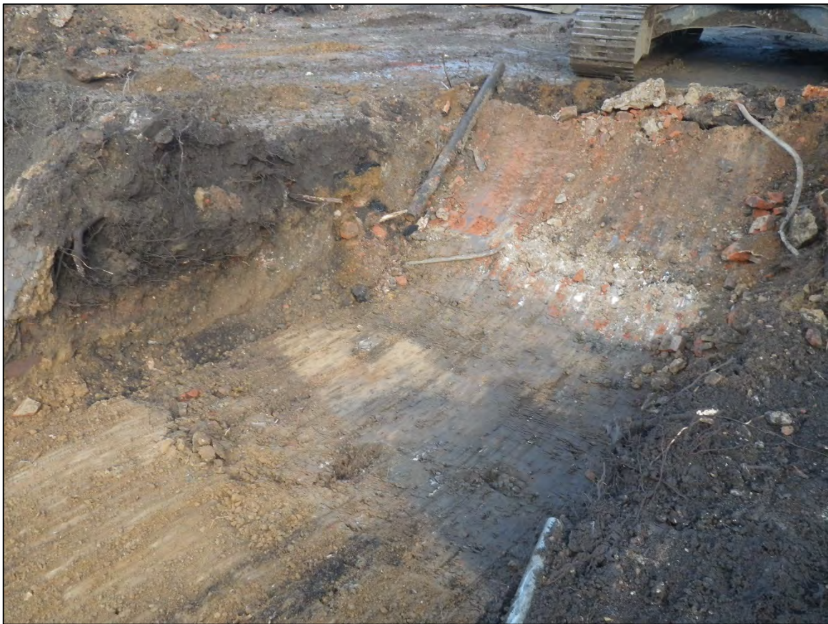
Plate 2. Contractors stripping site. Victorian wall and soil layer 0139 visible in section, with medieval pit 0145 exposed in base of excavation. Looking northeast
