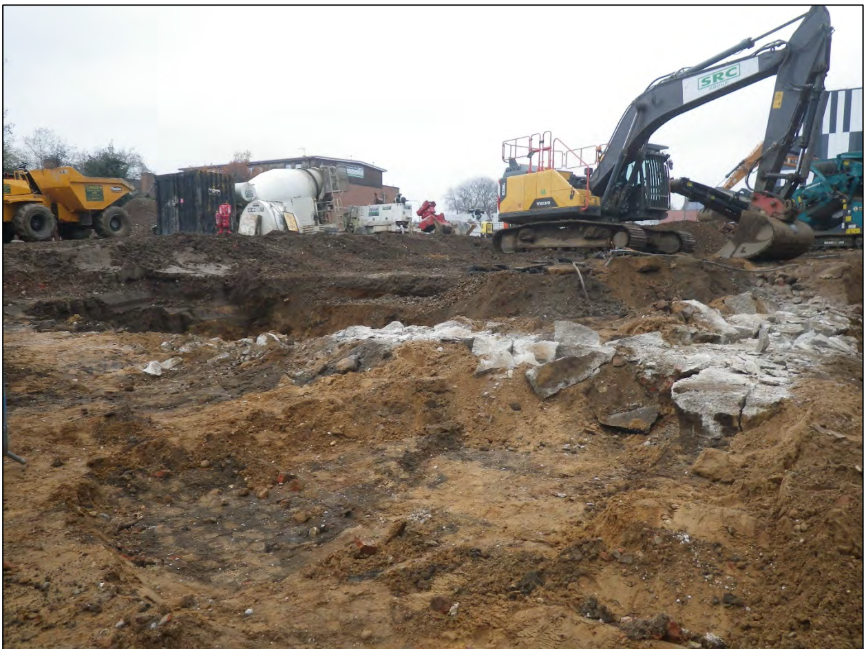
Plate 3. Contractors removing concrete footings in eastern half of site, with resultant damage. Looking northwest
