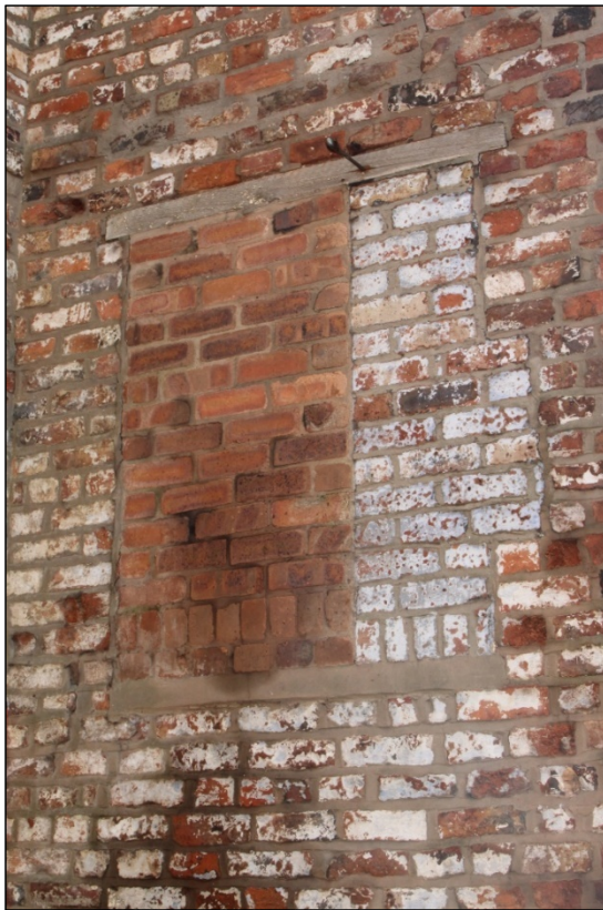
Photo 14: Detail of a blocked window opening within the southern elevation of the stair turret.
