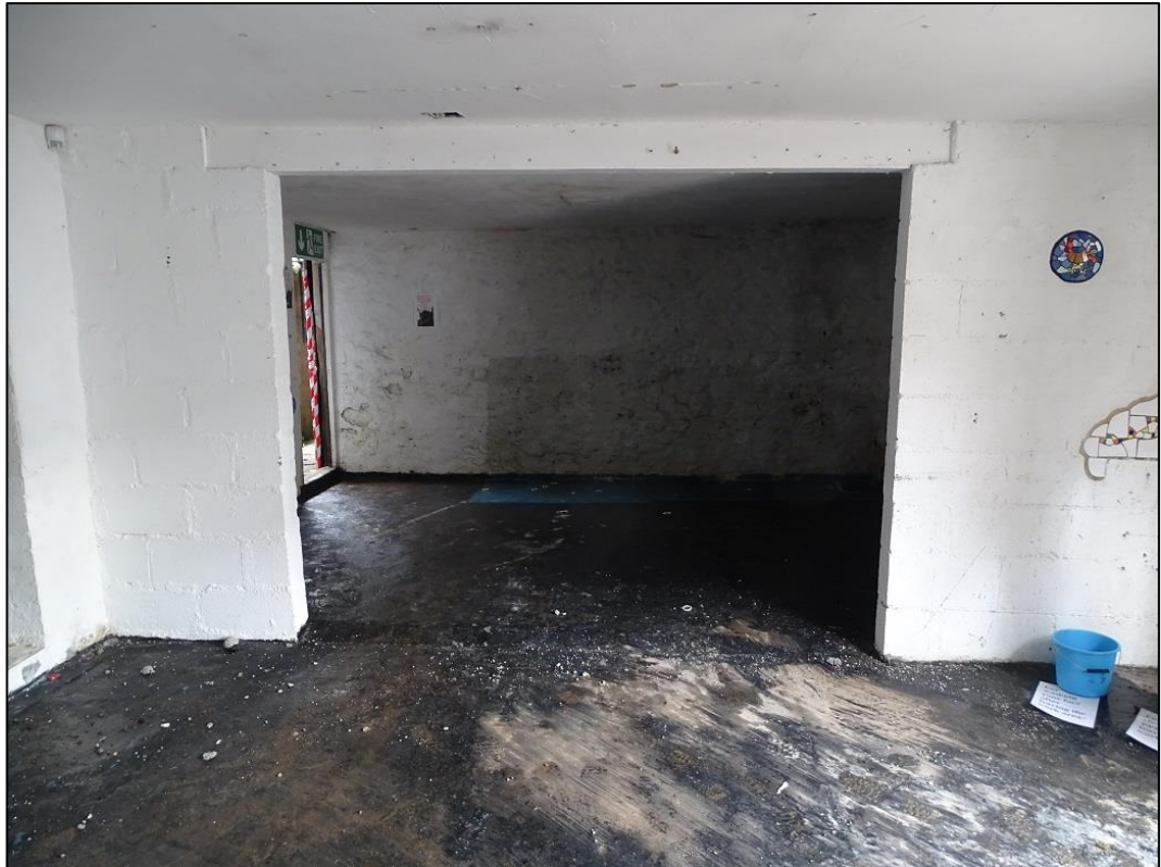
Photo 12: Interior of the Building at its ground floor south aspect looking north
