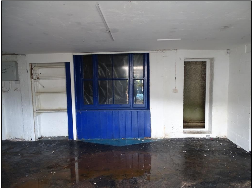
Photo 10: Interior of the Building at its ground floor south aspect looking west
