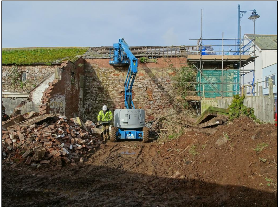
Photo 3: Exterior of the Building at its east elevation at ground floor north aspect looking west
