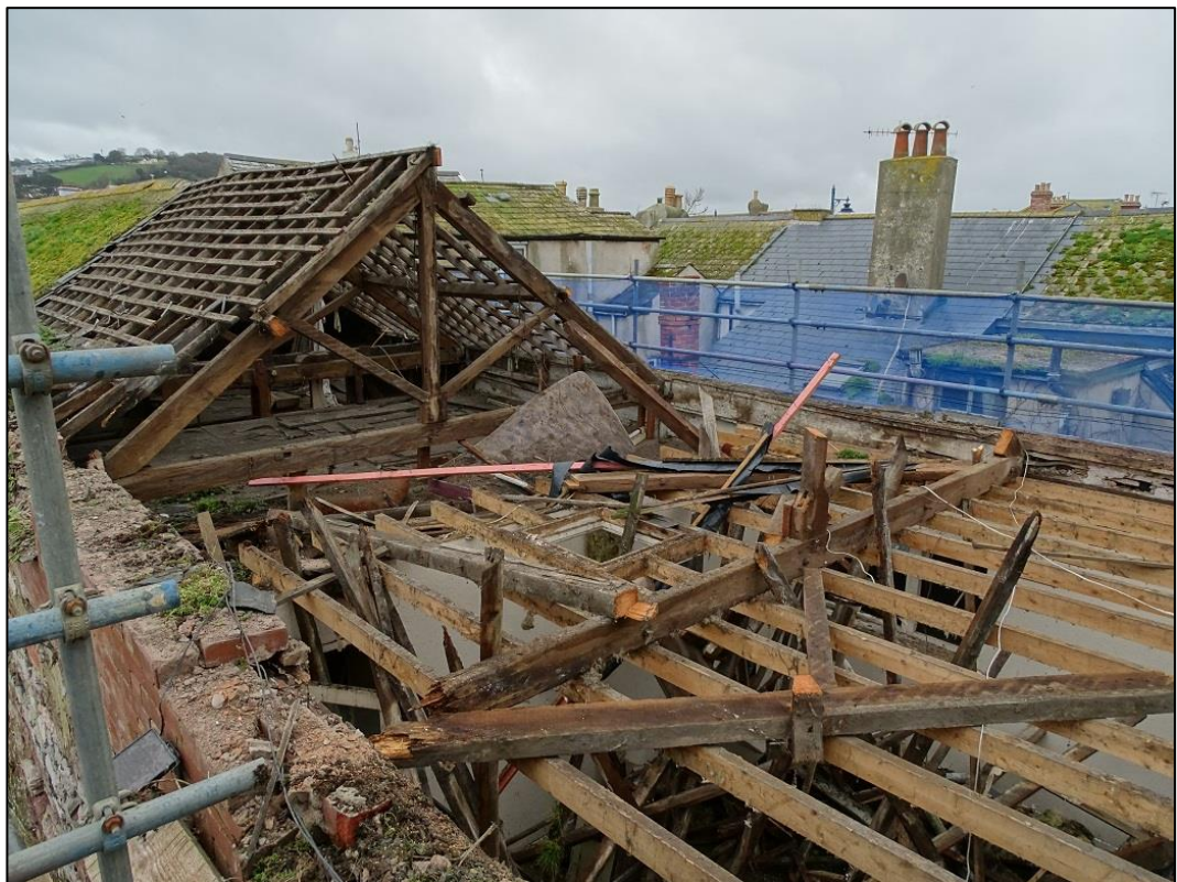
Photo 20: Demolition of the roof from the north elevation of the Building looking south west
