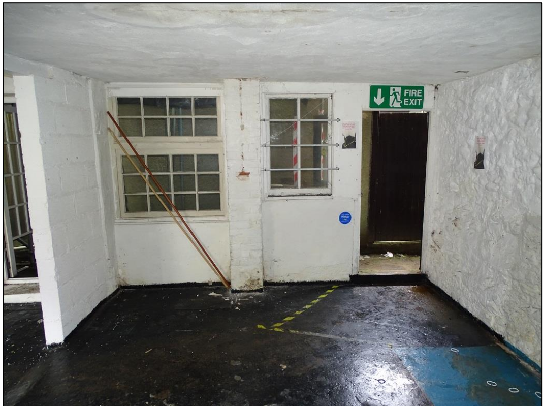
Photo 13: Interior of the Building at its ground floor south aspect looking west
