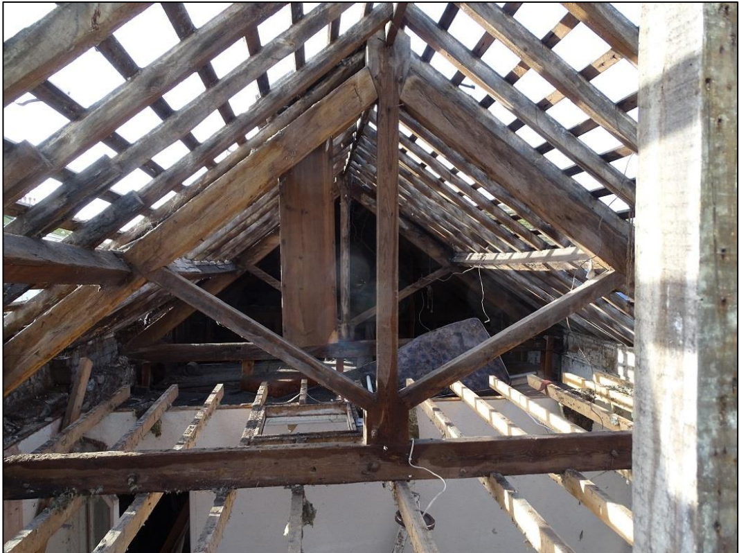
Photo 5: Exterior of the Building at its north elevation at roof level looking into the roof space
