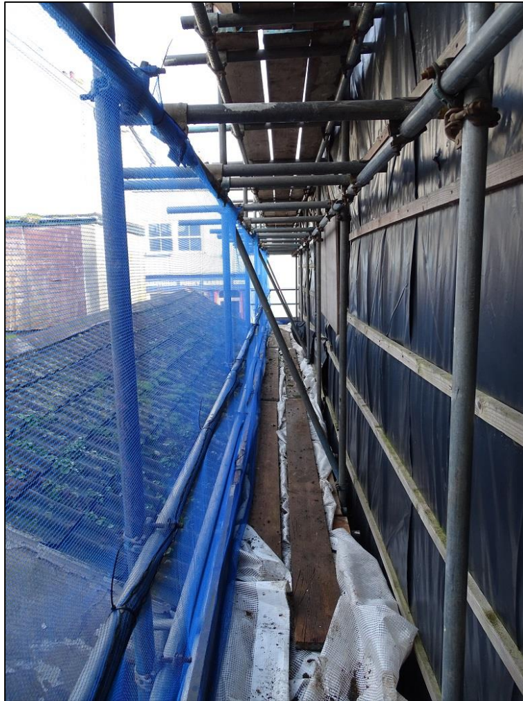
Photo 2: Exterior of the Building at its west elevation at first floor level looking north
