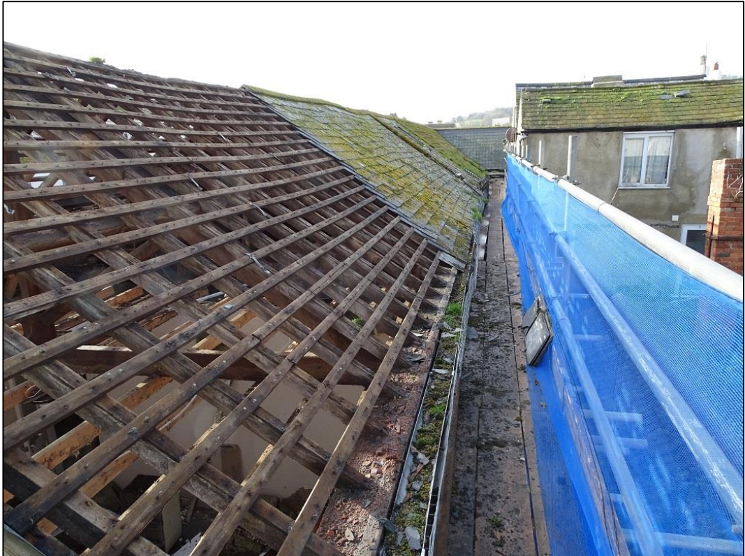
Photo 7: Exterior of the Building at its west elevation at roof level looking south
