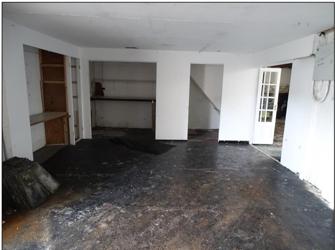
Photo 11: Interior of the Building at its ground floor south aspect looking south
