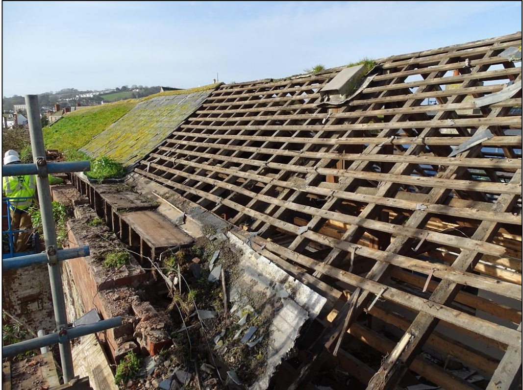
Photo 6: Exterior of the Building at its east elevation at roof level looking south
