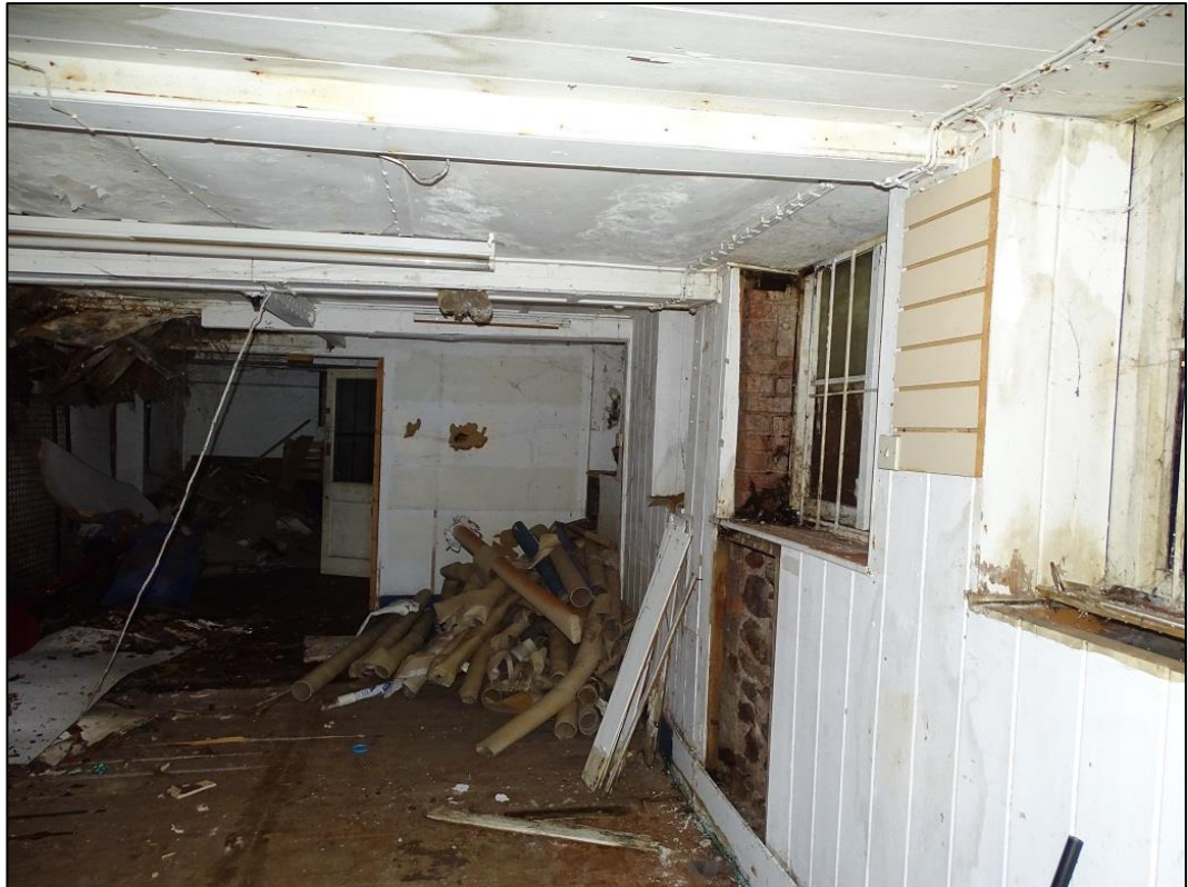
Photo 9: Interior of the Building at its ground floor north aspect looking south
