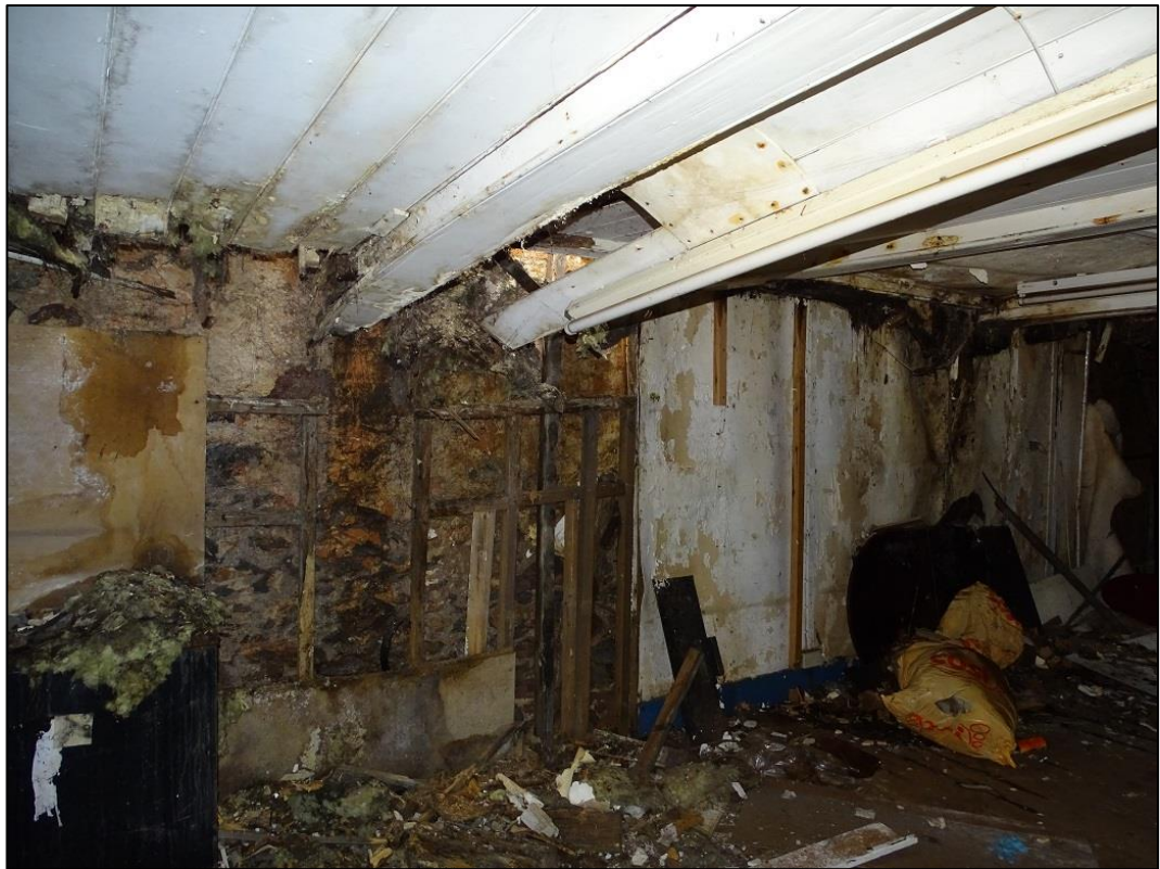
Photo 8: Interior of the Building at its ground floor north aspect looking east
