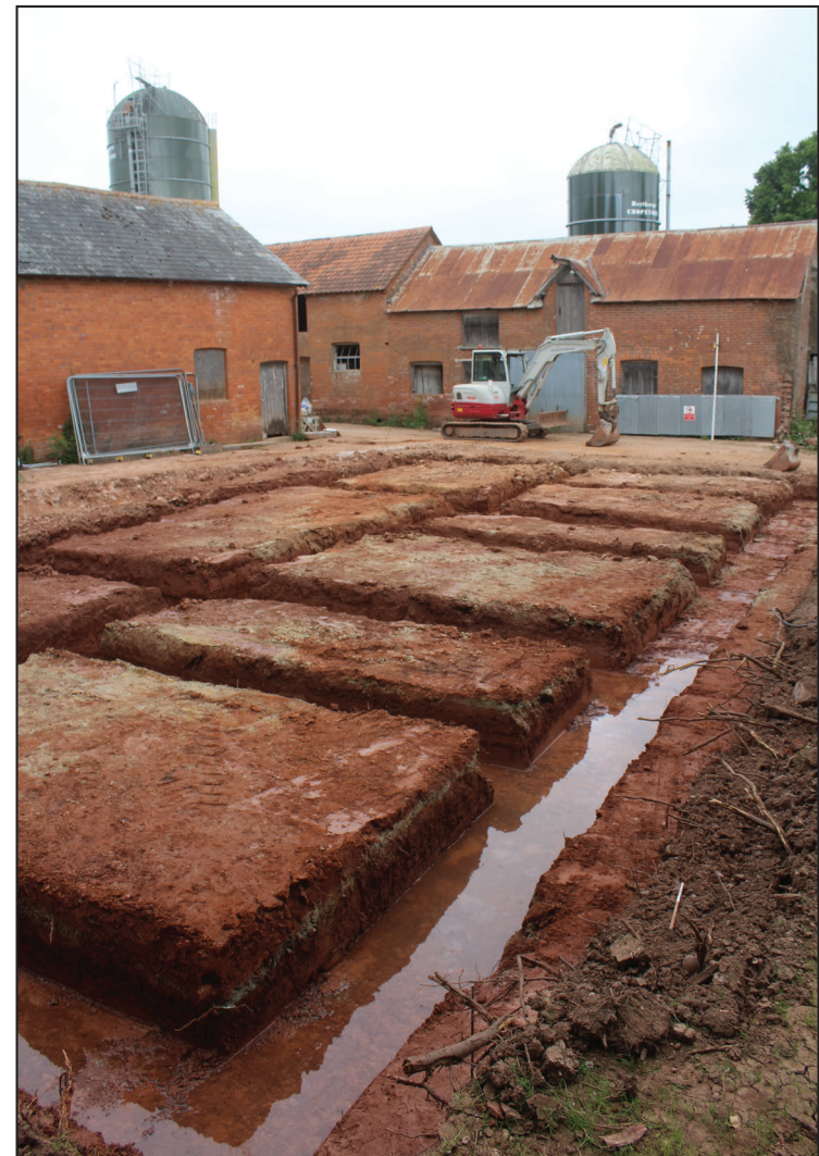
General shot of the excavated foundation trenches within the reduced footprint of the development, looking north-west
