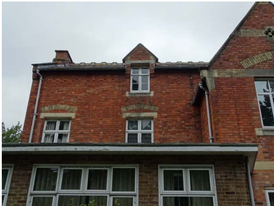
Photo 10: West elevation of the House at the north aspect above the 20th century extension
