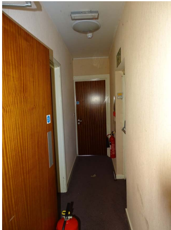
Photo 60: First floor north/south corridor of the House at north aspect looking north
