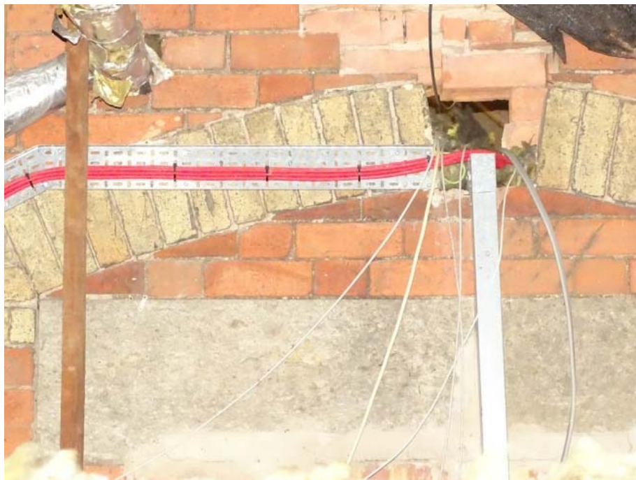
Photo 67: Looking west in attic space of 20th-century extension towards east elevation of the House detail
