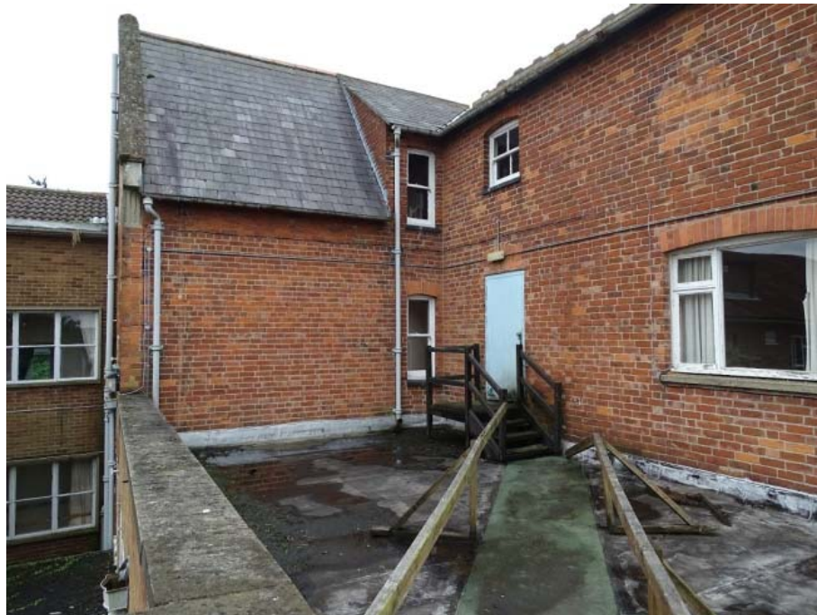
Photo 42: East elevation of the House from the flat roof of the north east 20th century extension
