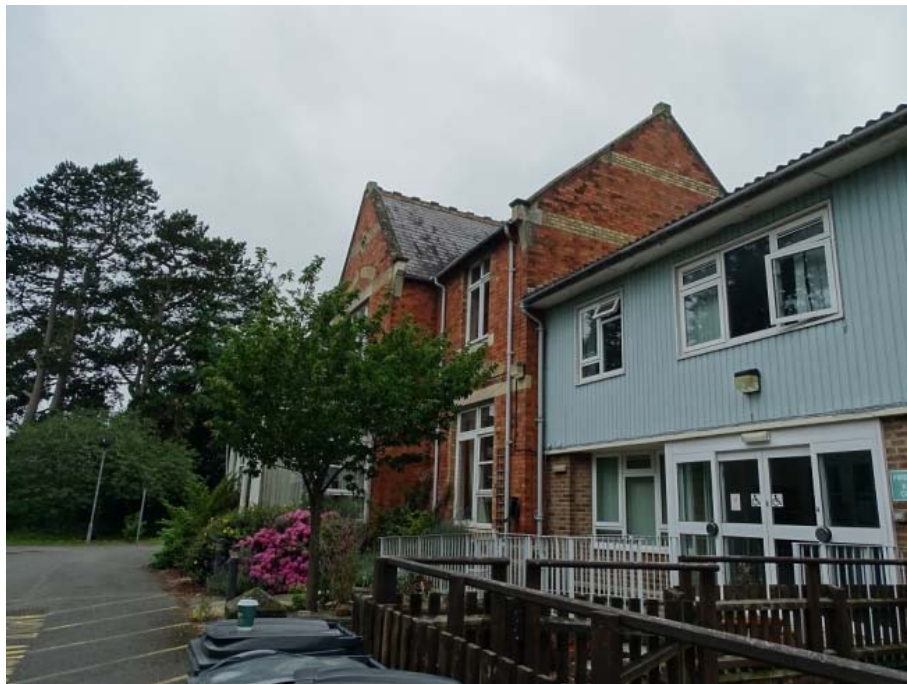
Photo 3: South elevation of the House interface with 20th century east aspect extension
