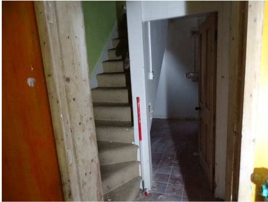
Photo 86: Cottages ground floor looking east to ground floor staircase at the west aspect
