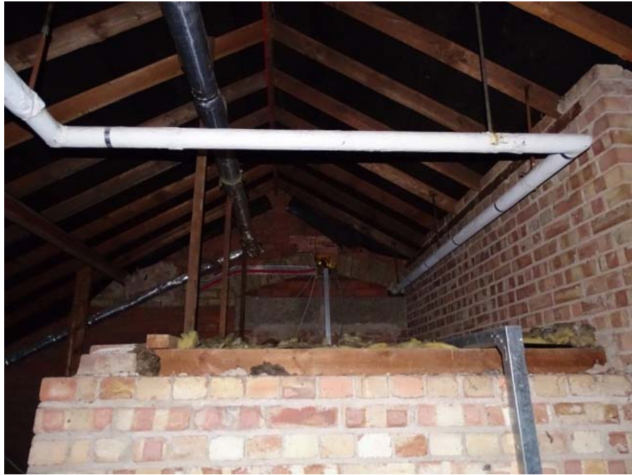
Photo 66: Looking west in attic space of 20th-century extension towards east elevation of the House
