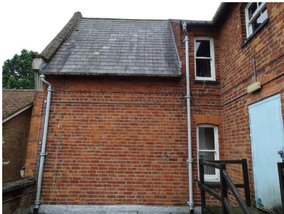
Photo 43: North elevation of the House at the east aspect from the north-east 20th century extension
