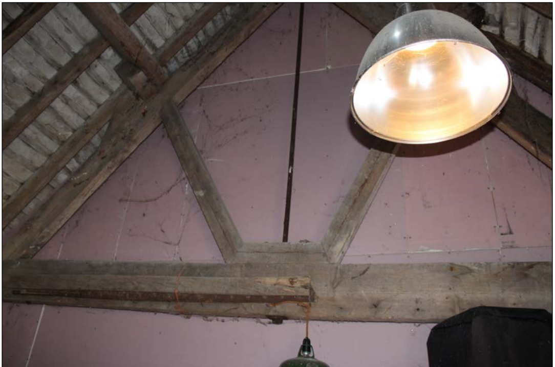
Fig. 31 King post 'without the king post' truss, southern end of the northern section
