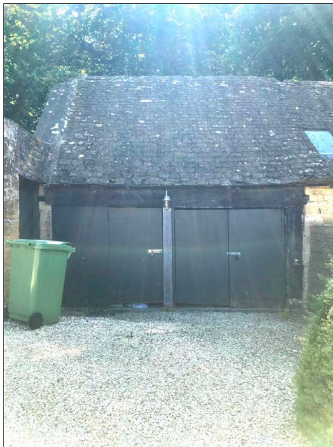
Fig. 28 View of garage doors, northern section of south garage, view to the east
