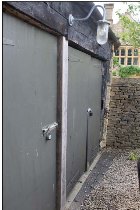
Fig. 41 Side view of northern section of south garage, view to the south
