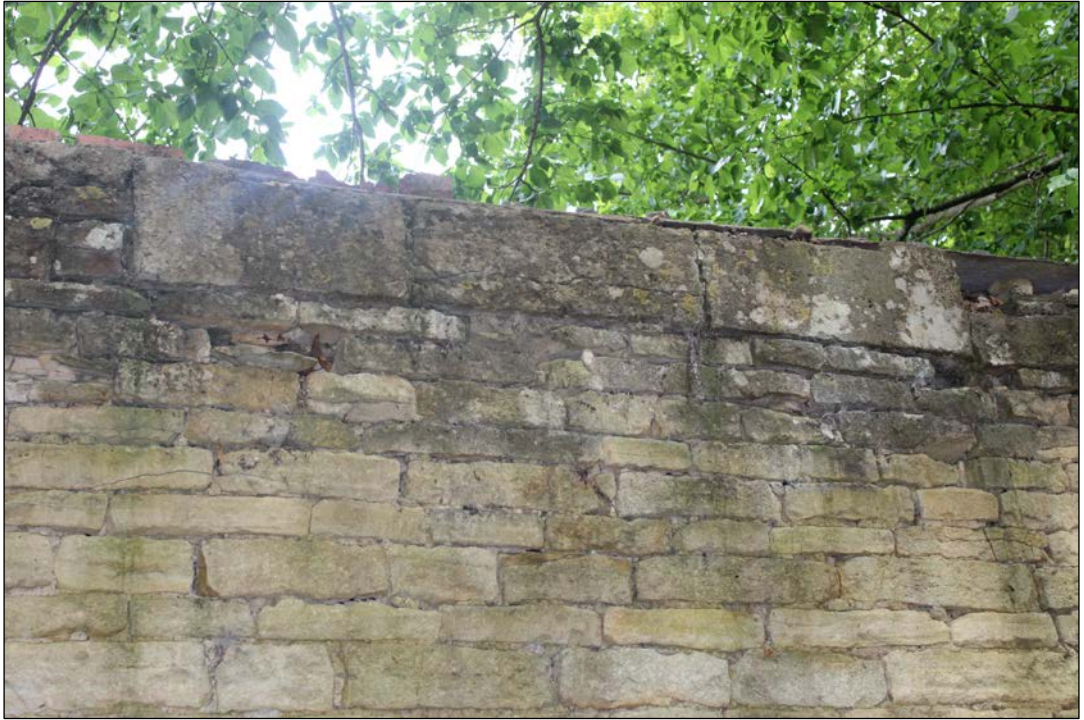
Fig.15 Truncated cill of window in the east elevation of the barn (now northern garage)
