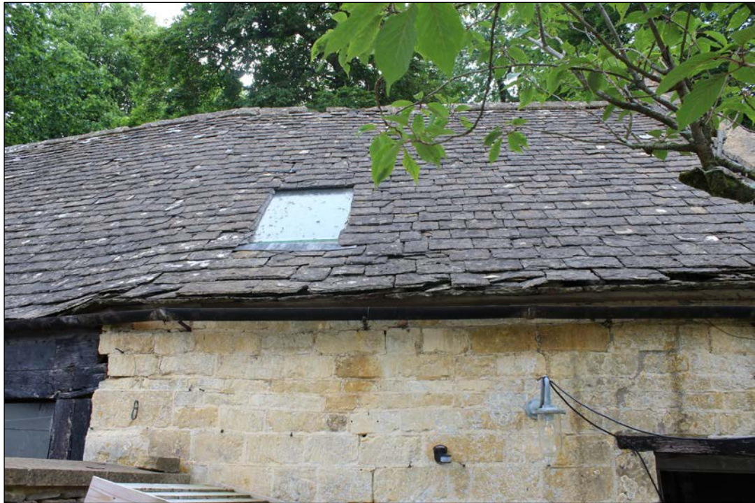
Fig.21 Section of roof, south garage, illustrating poor condition
