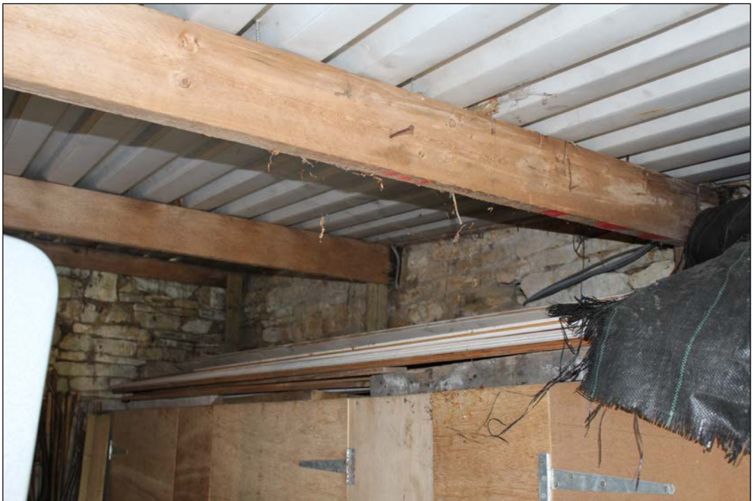
Fig.19 Interior of north garage, view to the south wall, obscured by storage cupboards
