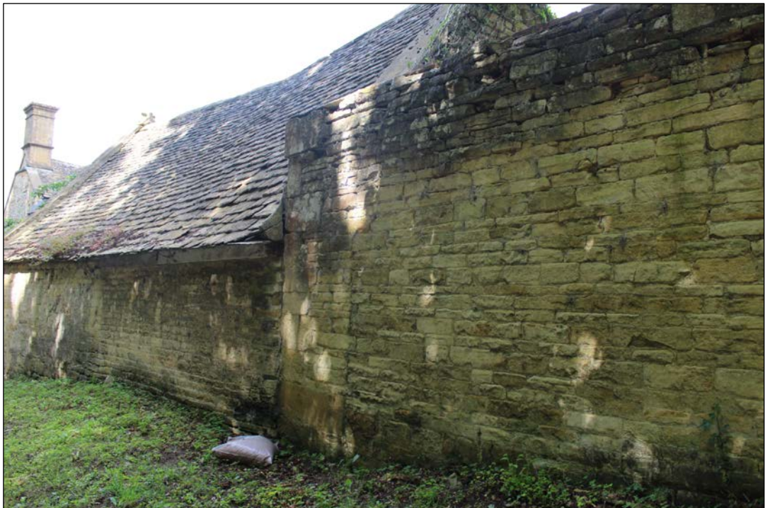
Fig. 27 External view of east wall of south garage, view to the south
