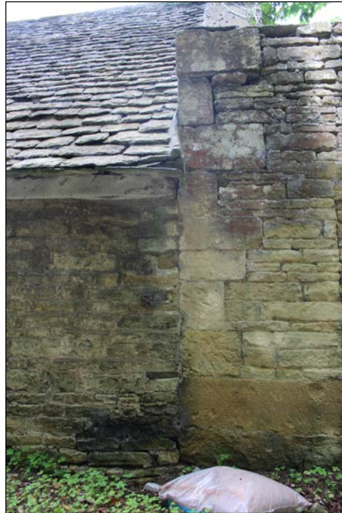
Fig. 35 Joint between south and north garages, viewed to the west from roadside
