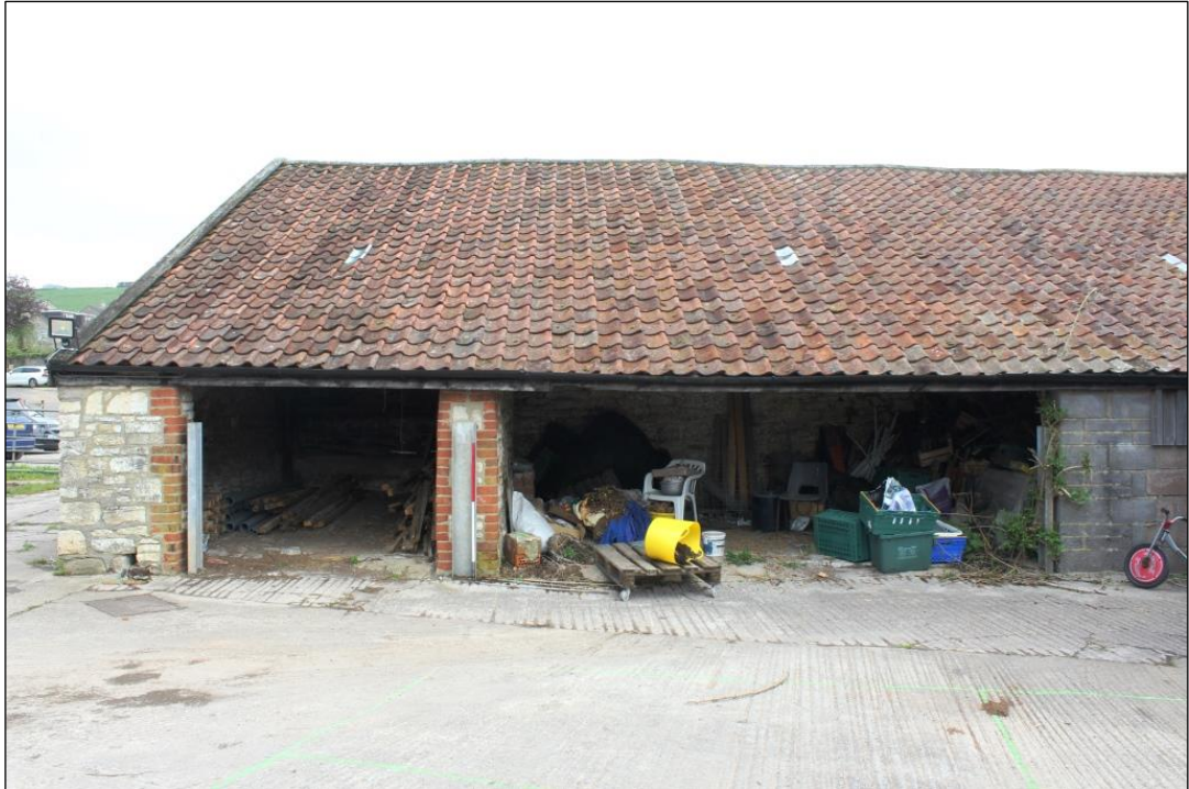
Photograph 13 Western extent of the south facing elevation of the stable and dairy block
