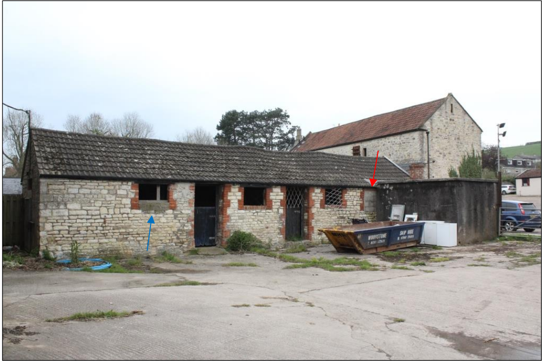
Photograph 3 East facing elevation of the bull pen and south facing elevation of the extension. The red arrow shows the blocked-in window and the blue arrow the concrete base of window
