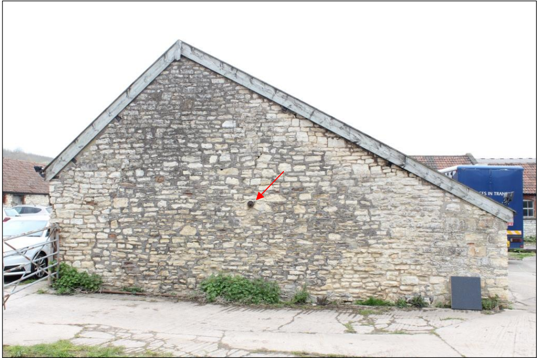
Photograph 12 West elevation of the stable and dairy block. Red arrow shows metal plate
