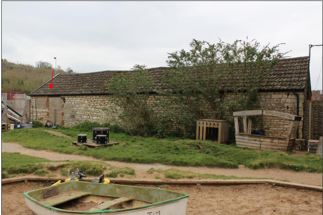
Photograph 5 West elevation of the bull pen. Red arrow shows the blocked-in window and door
