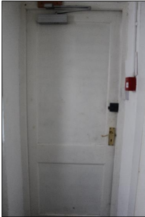
Photo 25: Detail of door opening within the northern elevation of the Boiler Room.
