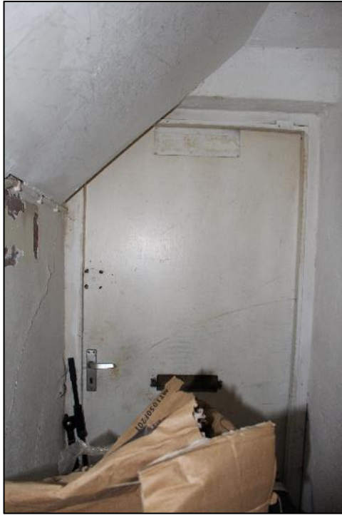
Photo 26: Door opening within the northern elevation of the late 18th/early 19th century range.
