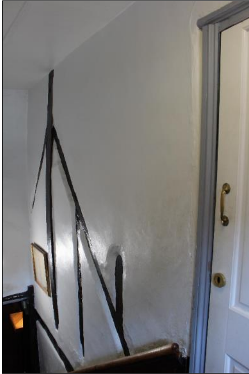
Photo 63: Detail of exposed timber framing/ roof truss within the northern wall of the stairwell.
