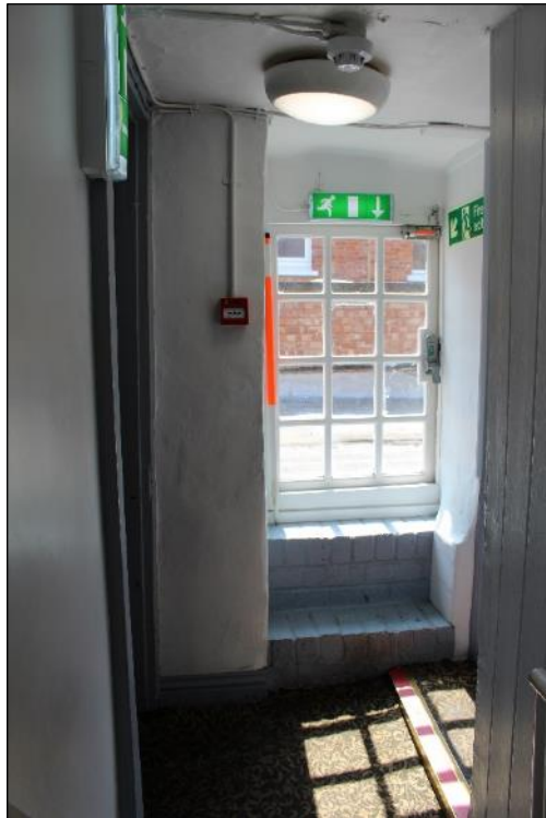
Photo 73: External window/door opening leading on to the flat roof of the 20th-century building.
