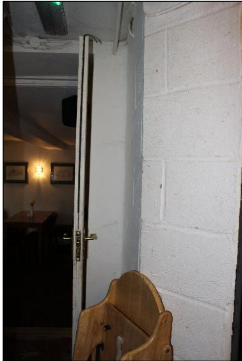
Photo 28: Breeze block wall construction to the southern wall of the Staff WC/Store.
