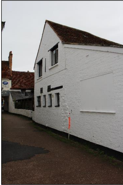
Photo 8: The re-built brick gable end of the late 18th/early 19th century range.
