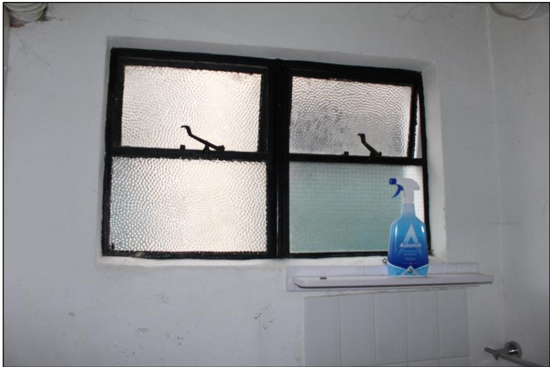
Photo 24: Detail of window opening within the western elevation of the Boiler Room.
