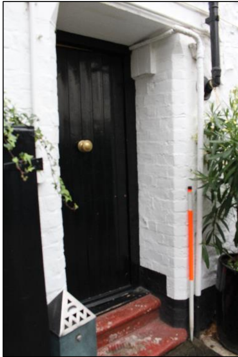
Photo 6: Detail of stop chamfer door opening within the 18th/early 19th century range.
