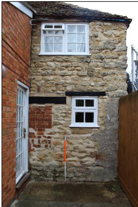
Photo 11: Detail of the southern elevation of the late 18th/early 19th century range.
