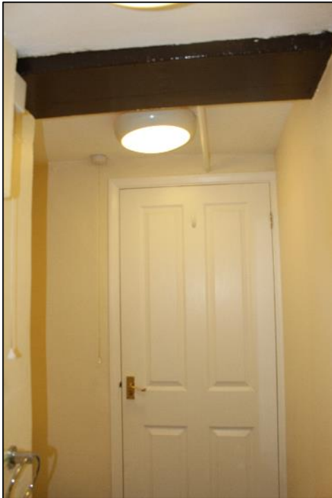
Photo 37: Detail of boxed timber and door opening within the en-suite bathroom of Room 7.
