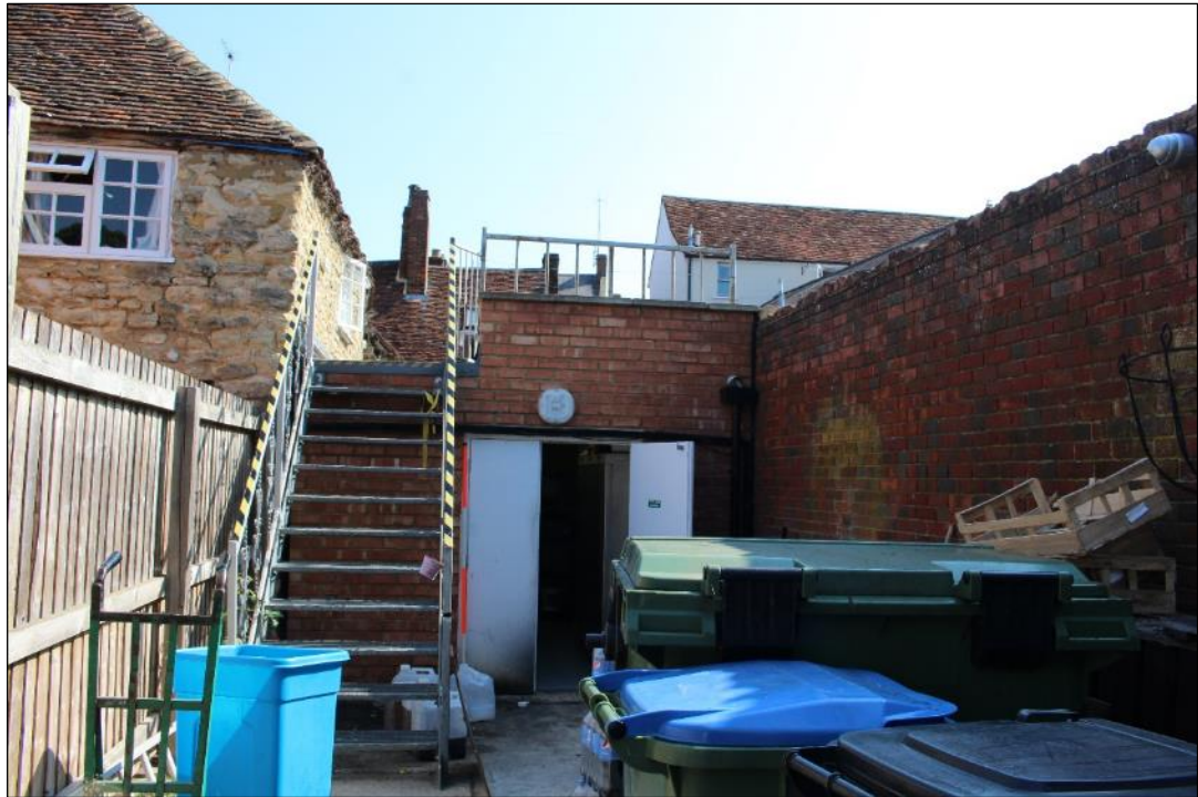
Photo 47: The southern elevation of the late 20th century kitchen extension and the late 18th/early 19th century subsidiary building.
